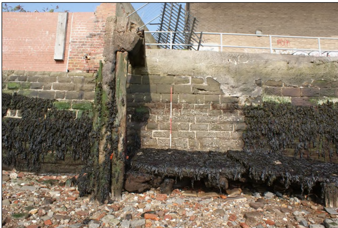
Plate 9: ESE facing elevation of NNE-SSW aligned quayside wall showing collapsed ramp in the foreground, View WNW, 2m scale.
