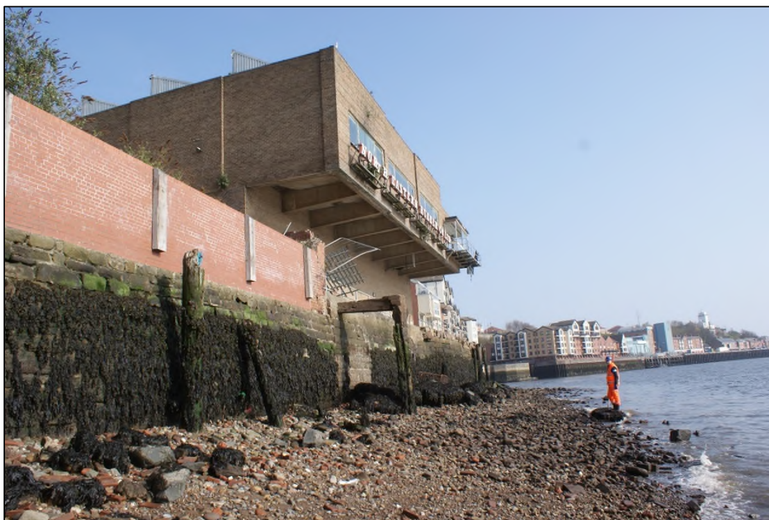
Plate 10: Oblique view of NNE-SSW aligned quayside wall showing collapsed ramp, View north, 2m scale.
