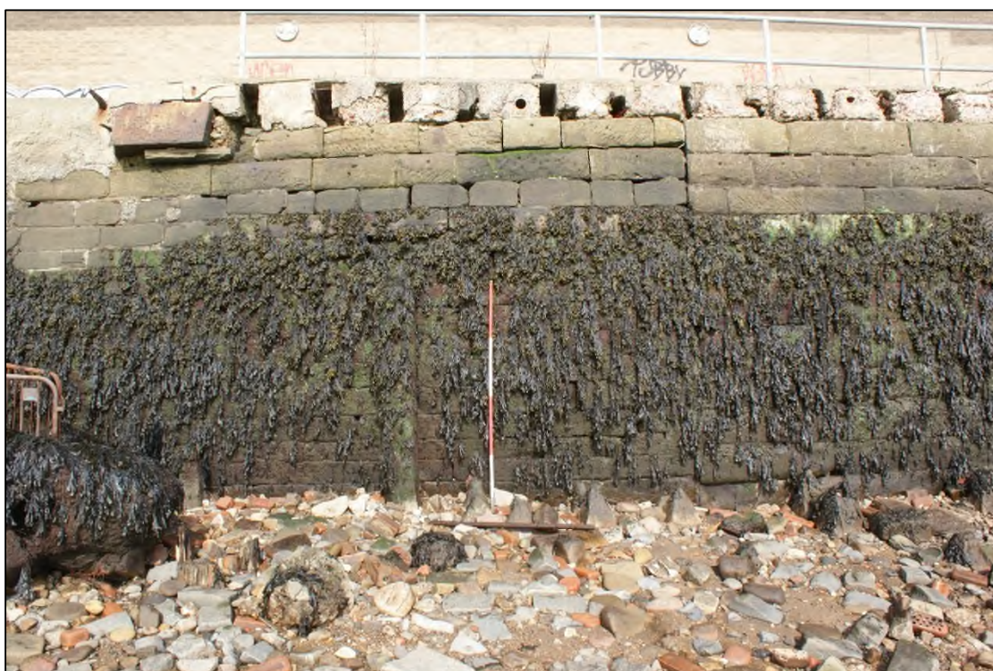
Plate 6: ESE facing elevation of NNE-SSW aligned quayside wall showing timber mooring, View WNW, 2m scale.
