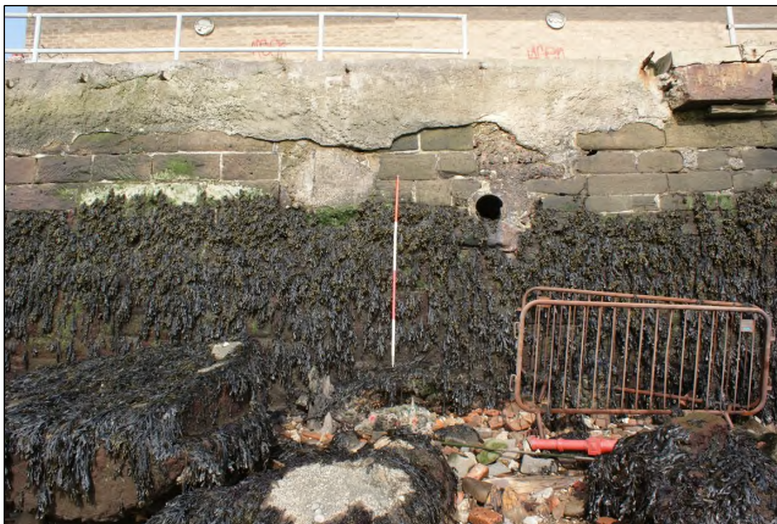
Plate 7: ESE facing elevation of NNE-SSW aligned quayside wall showing concrete render to and drain, View WNW, 2m scale.
