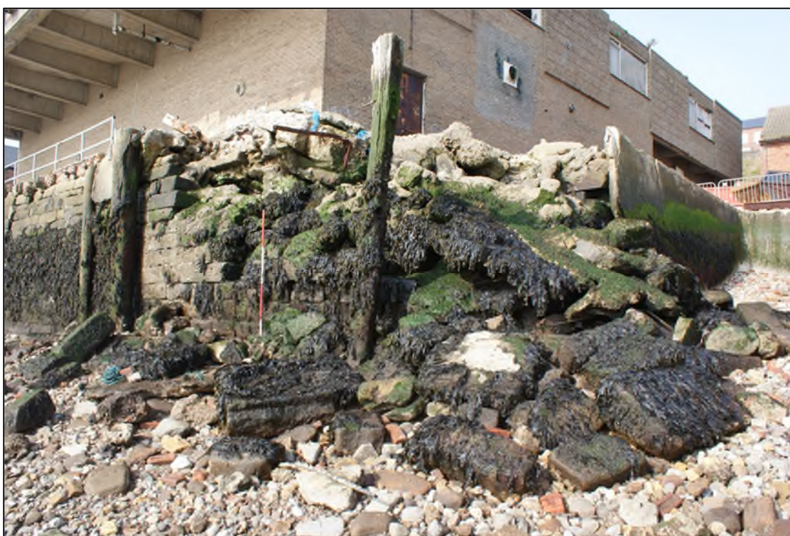
Plate 2: North-eastern corner of collapsed quayside wall, view south-west, 2m scale.
