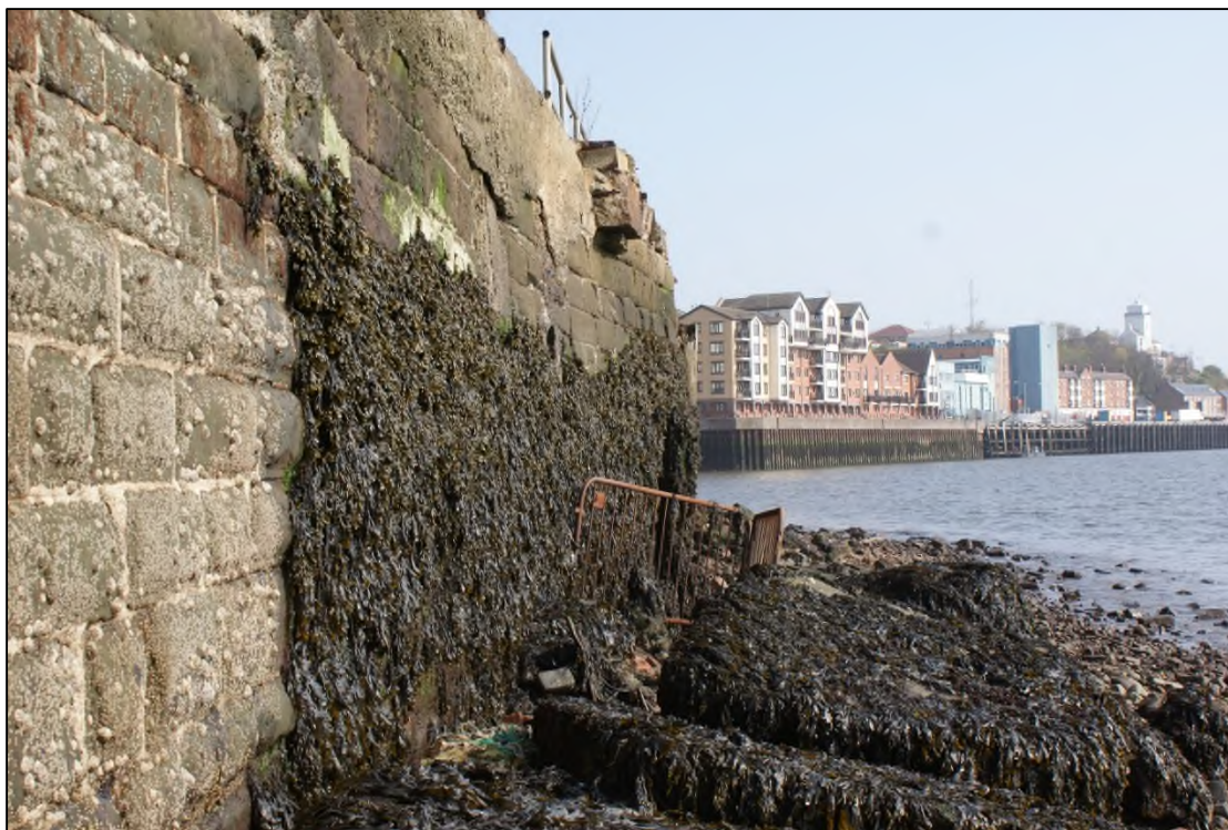
Plate 11: Oblique view of NNE-SSW aligned quayside wall showing area of bulging, View north.
