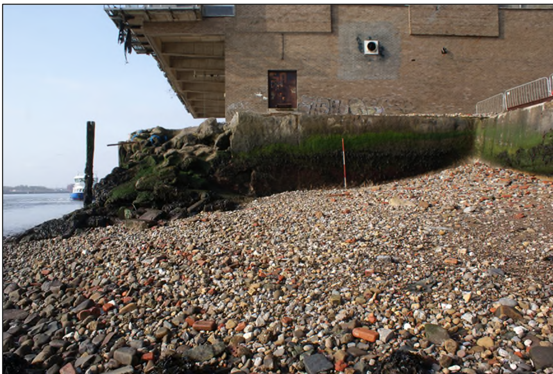
Plate 1: NNE facing elevation of WNW-ESE aligned quayside wall, view SSW, 2m scale.
