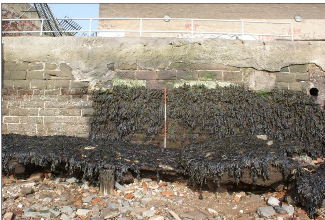
Plate 8: ESE facing elevation of NNE-SSW aligned quayside wall showing collapsed concrete surface in the foreground, View WNW, 2m scale.
