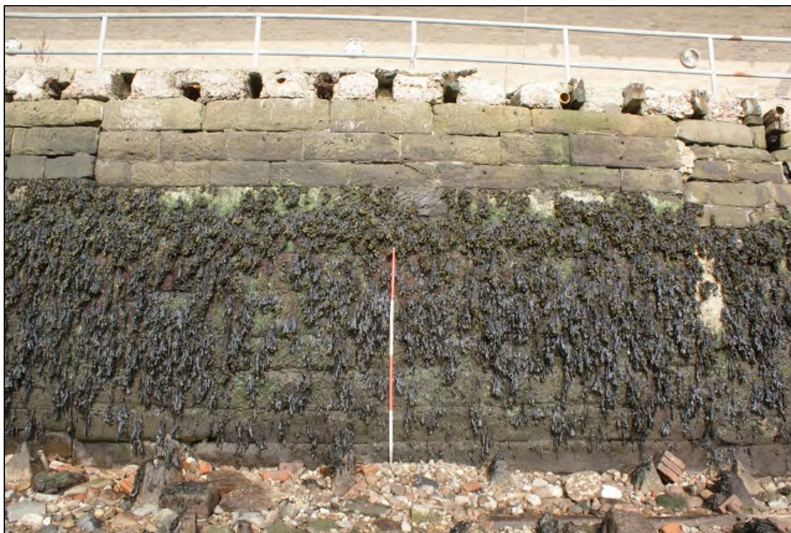
Plate 5: ESE facing elevation of NNE-SSW aligned quayside wall showing area of masonry infill, View WNW, 2m scale.
