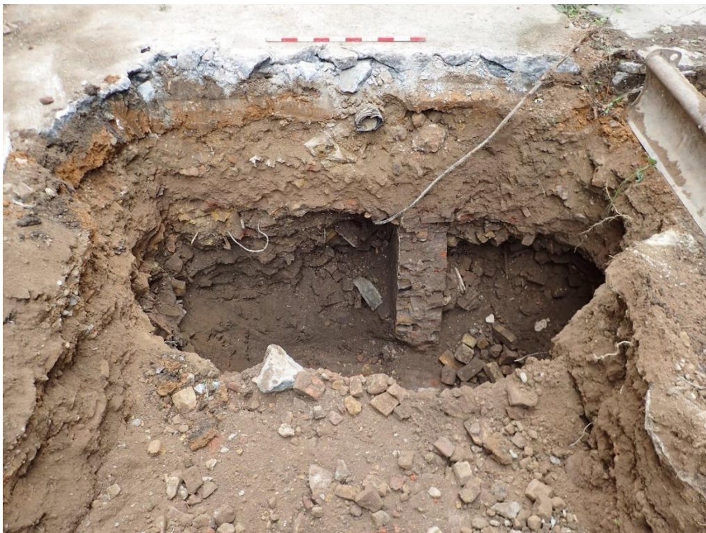
Plate 14: Trench 3, looking south, basement wall [102] with backfill deposit [100] and [101] overlain by layer [99]
