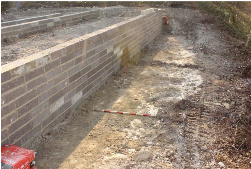
Plate 1 View to the south of exposed made ground - on top of the embankment
