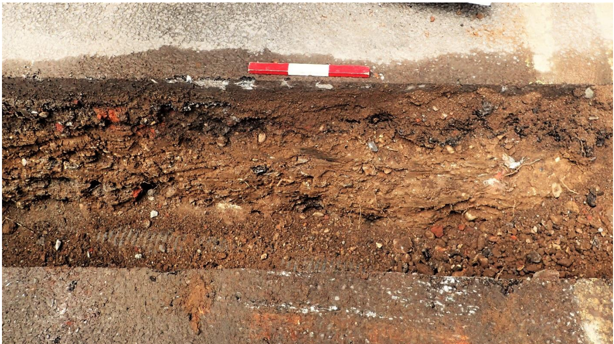
Plate 9: Trench 3, Section 5, view to north-west, scale 0.30m. Made ground and black plastic conduit containing live electrical services.
