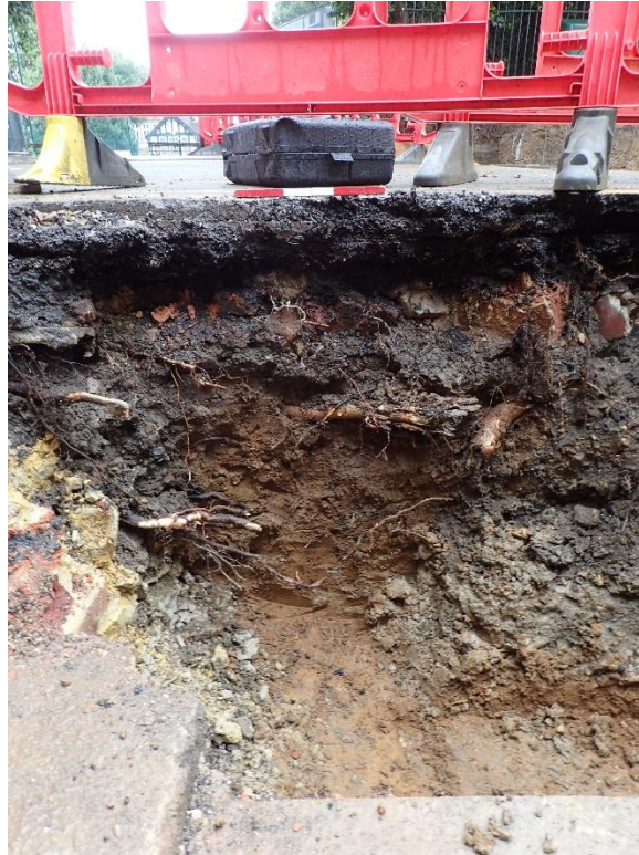
Plate 12: Trench 6, Section 9, view to north-west, scale 0.30m. Made ground and truncated brickearth [31].
