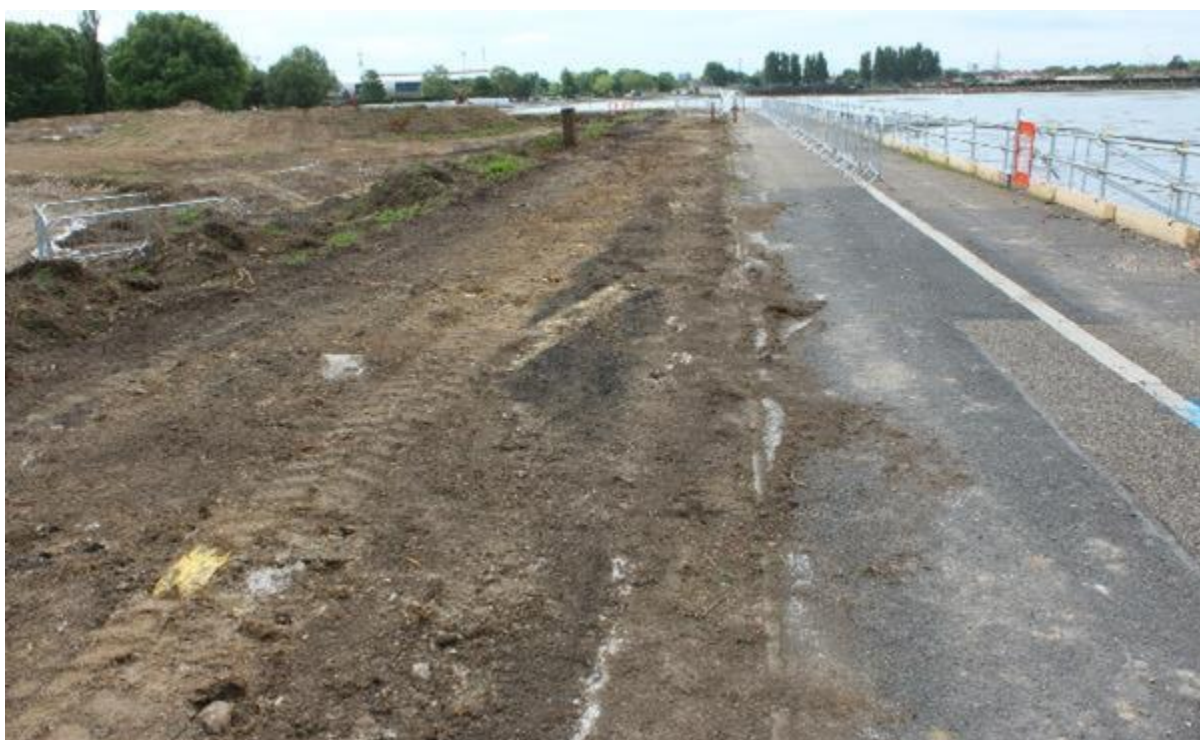
Plate 2. Southwest facing shot of stripped area behind Sea wall, Zone 1.
