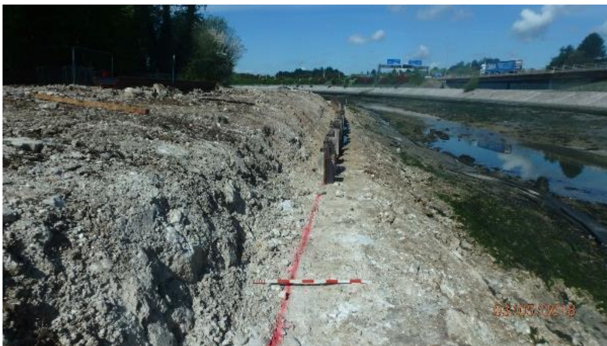
Plate 9. West facing shot of ground works at the northern end of Zone 2.
