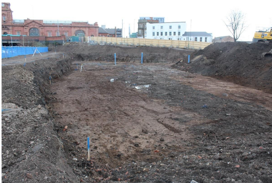
Plate 4: Northern half of monitored area looking east, excavated to maximum depth, brown deposit at base is (017), radiocarbon dated to the Middle Bronze-Age
