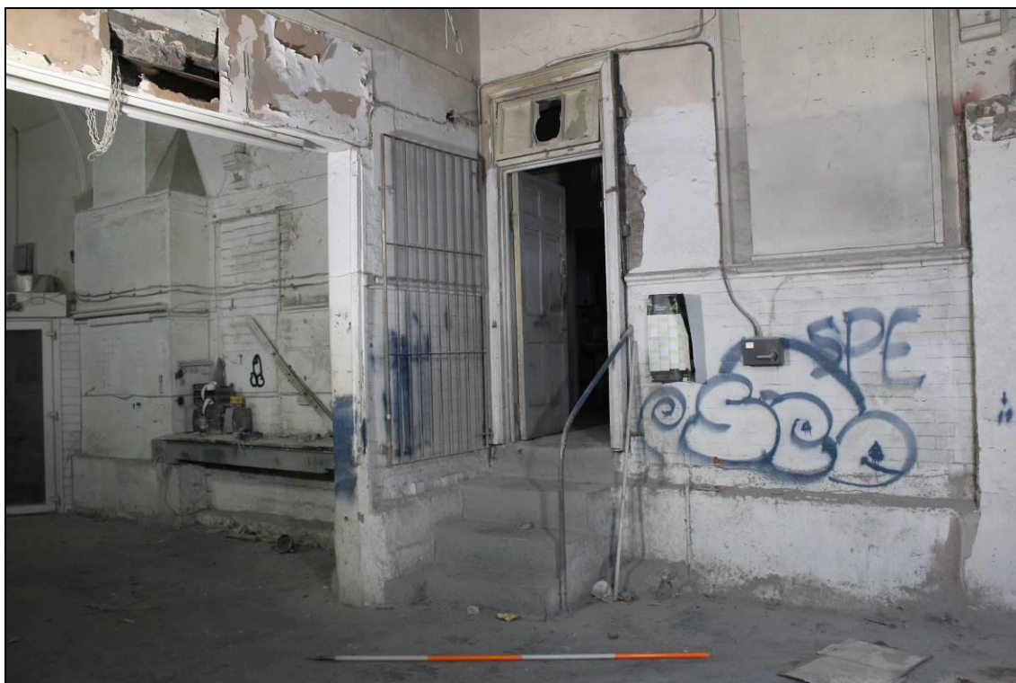
Plate 35: Room 1b, doorway and modern addition of concrete steps: view southwest, scale: 2m
