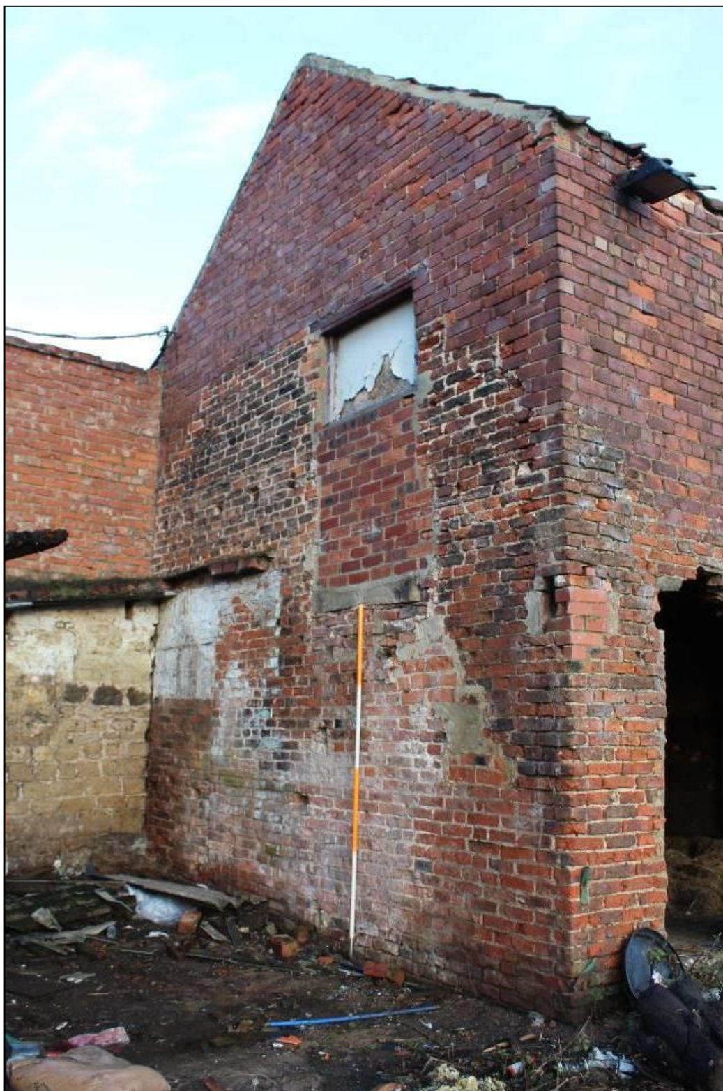
Plate 42: South facing elevation of Building C1 showing blocked up doorway (ground floor) and pitching hole (first floor): view northwest, 2m scale
