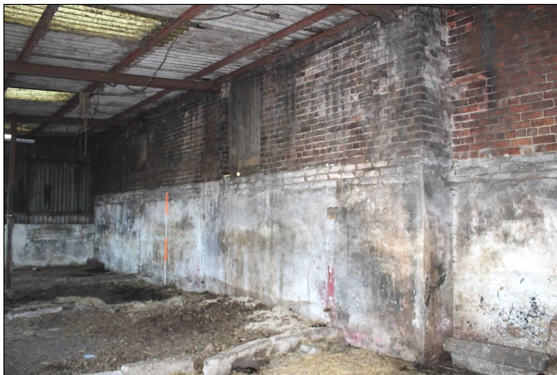
Plate 48: Building C2, western elevation (taken from inside Building C4; note blocked up pitching hole and window on first floor): view northeast, 2m scale
