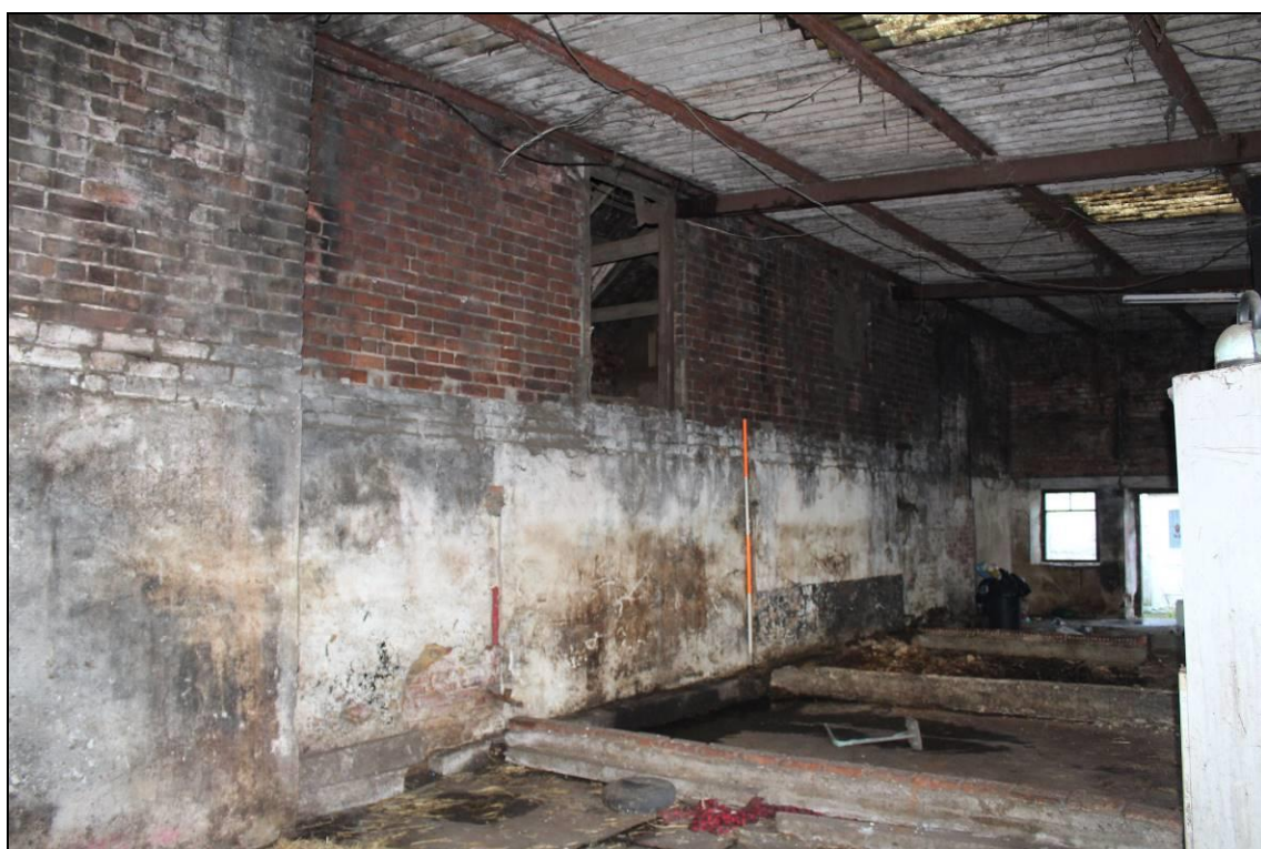
Plate 44: Building C1 western elevation (taken from inside Building C4). Note first floor pitching hole into hay loft: view southeast, 2m scale
