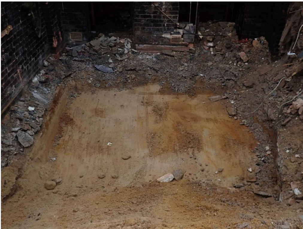
Figure 1 Looking north - showing natural sands below the previous location of the basement slab
