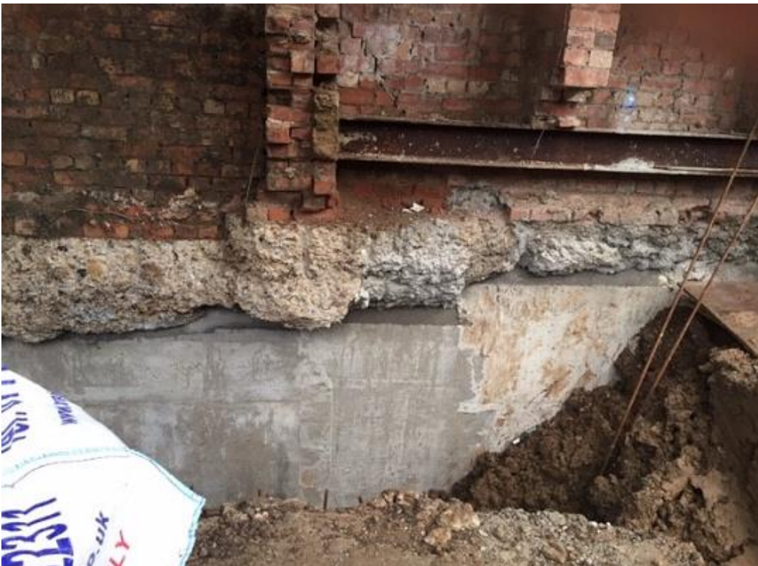
Plate 2: View to south of underpinning along central southern boundary illustrating depth of terrace foundations
