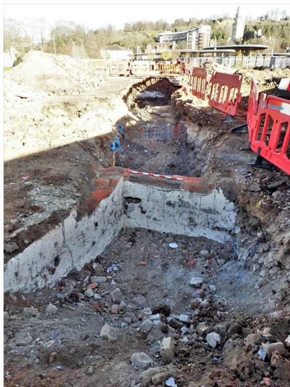
Plate 15: Trench 12, view to north-east, scale 1m. Interior walls [78] of Building 5, the cellar of the public house.
