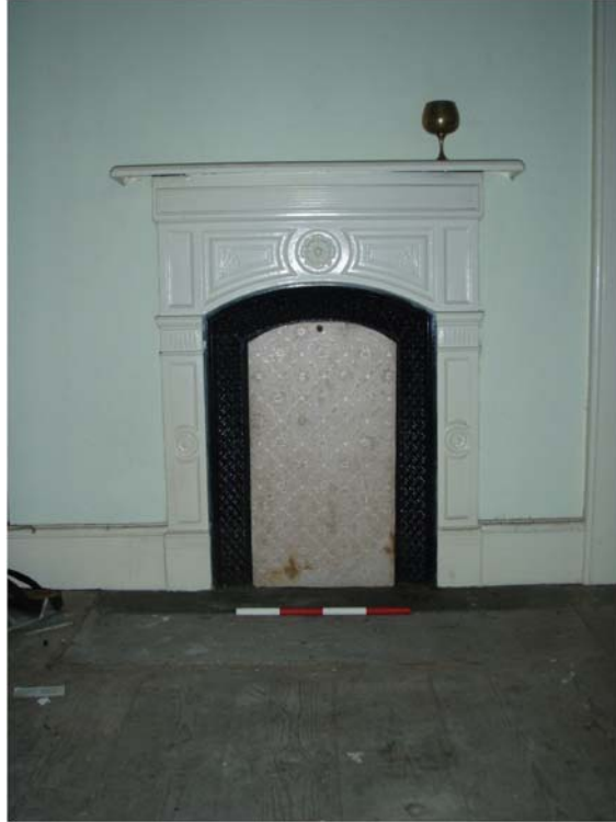
Plate 14 Original fireplace in west wall of north-east bedroom, looking west. Scale 5x100mm
