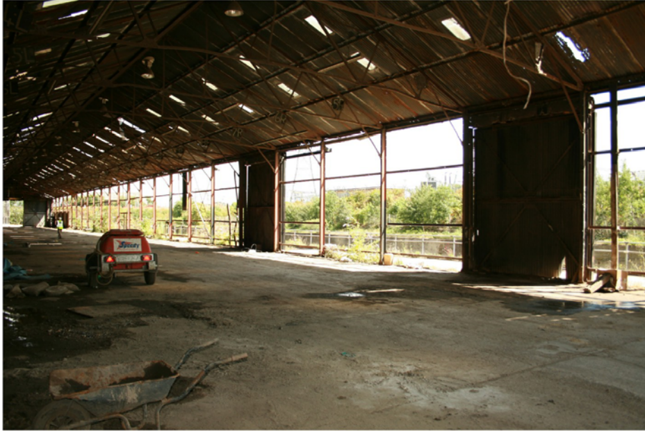
Plate 5 Internal view of east wall of Shed 1 looking north-east, showing two double vehicular access doors towards southern end
