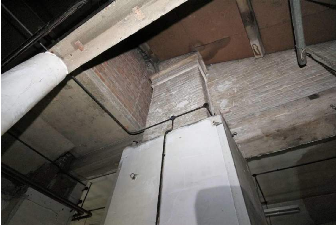
Plate 13 Former western elevation to (A), showing arch, pier and later concrete stair, looking east
