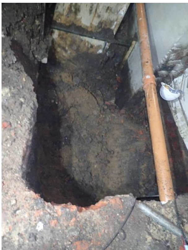
Plate 1: Disturbed natural close to the base of the sequence in Test Pit 26 (Group 2), which could represent the base of an agricultural horizon. Photograph faces west
