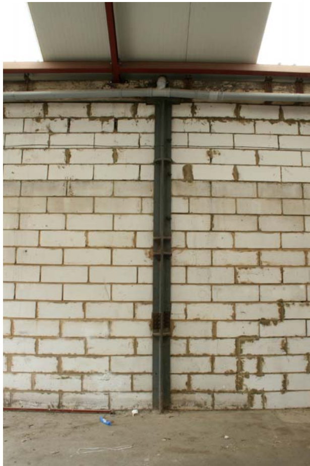
Plate 20 Detail of 19 th -century cruciform cast iron stanchions supporting timber beam in central bay of Building 2, looking south-east
