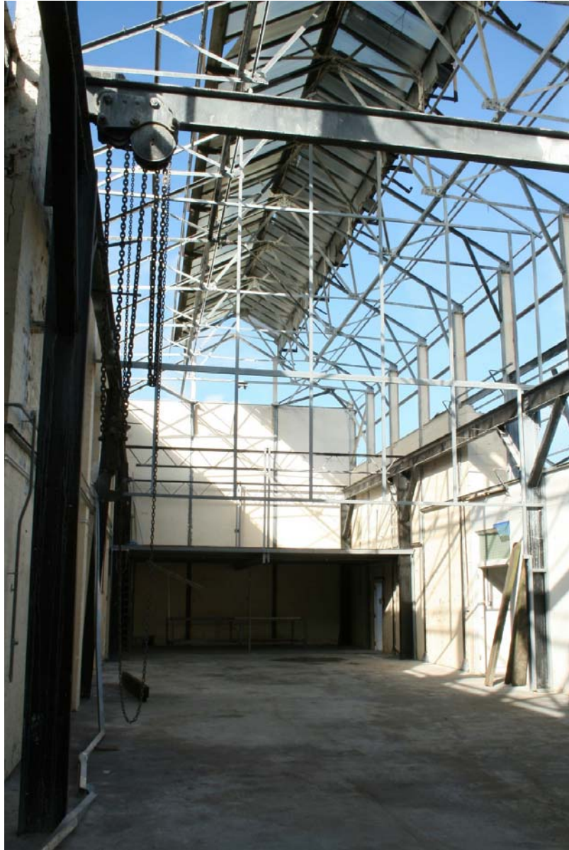
Plate 12 Internal view of Building 1 showing detail of lifting tackle and frame, looking north-east
