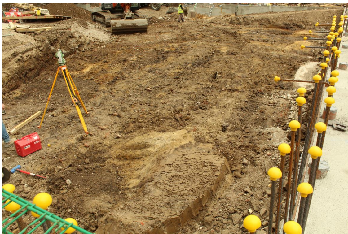
Plate 3: view west area of Trench 3 showing (foreground) a small 'island' of untruncated natural sealed by [124]. Looking north-west.
