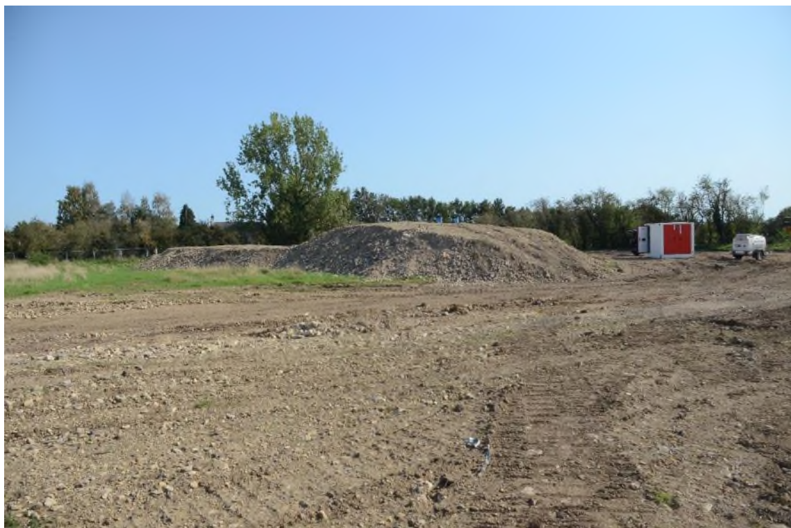
Plate 1: The demolition rubble containing asbestos in the northern field, view east
