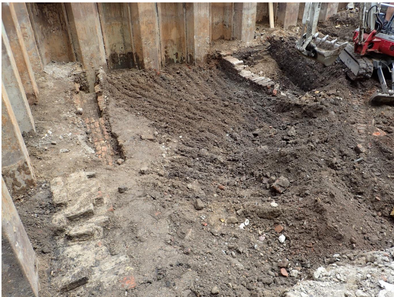
Plate 4: Overview of site, showing brick lined culvert and brick lined pit. Looking east.
