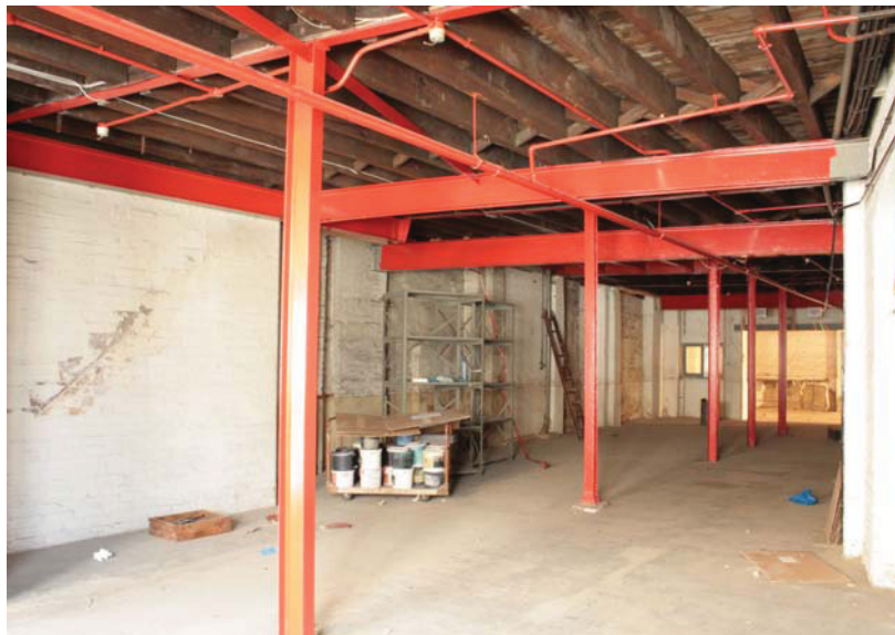
Plate 11 Internal view of Building 2, showing general layout of ground floor and the I-section stanchion frame, looking south
