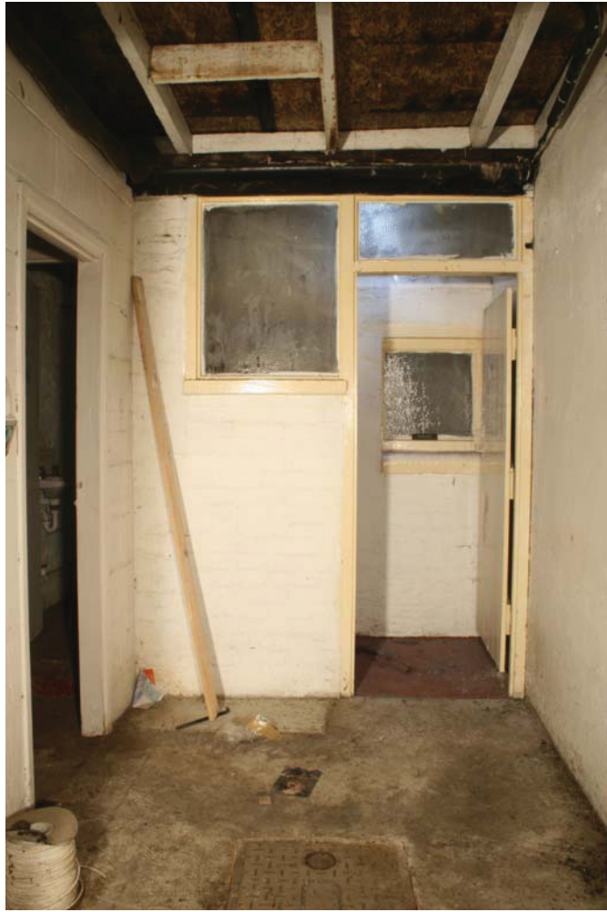
Plate 15 Internal view of Building 3, showing temporary roofed area with WC, looking south-west
