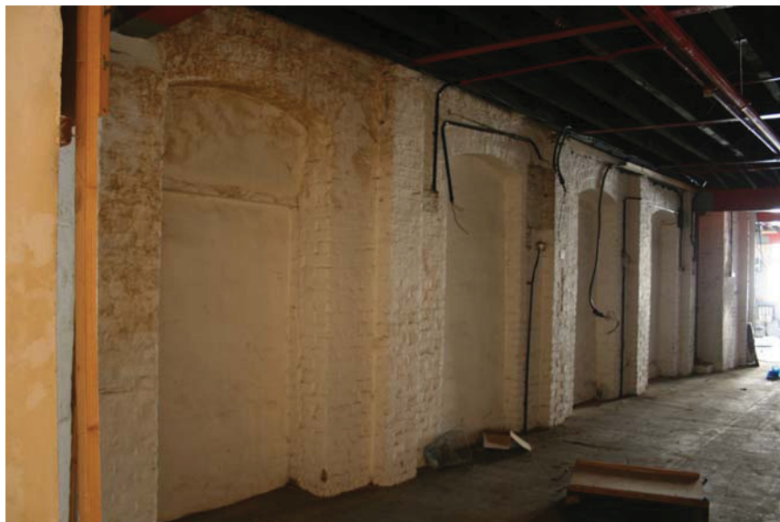
Plate 10 Internal view of Building 2, showing blocked segmental headed arches on ground floor, looking north
