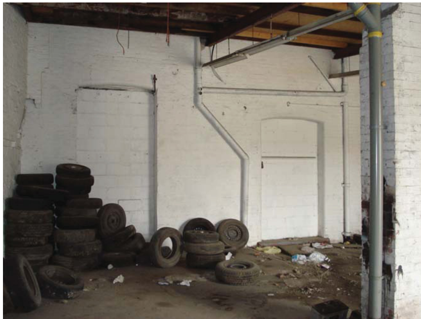
Plate 22 Internal view of Building 5, showing blockings on the adjoining wall of Building 4, looking north-east
