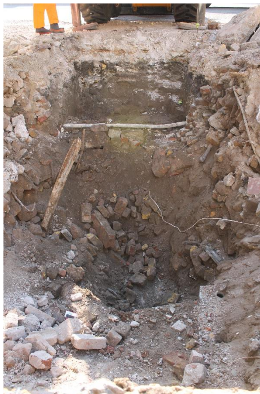
Plate 4. Sondage completed in Trench 3 through demolition layer [7], showing concrete surface [18] (looking east).
