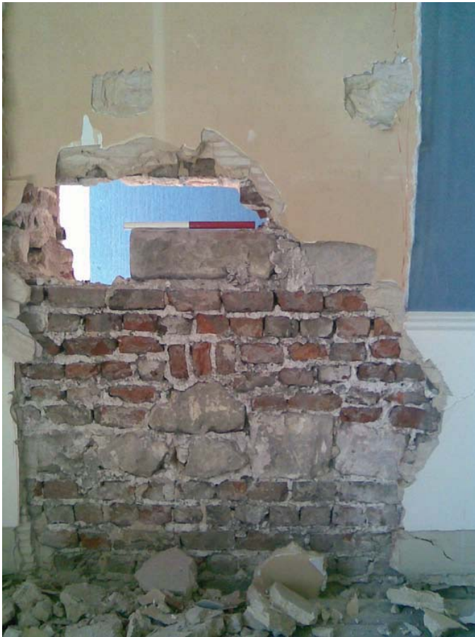
Plate 8. Second Floor, bedroom 6, wall[12]. Scale is 0.40m
