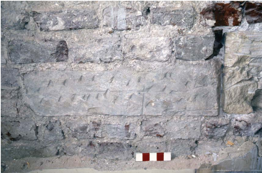
Plate 5. Second Floor, North bathroom. Close up of worked stone, Scale is 10cm
