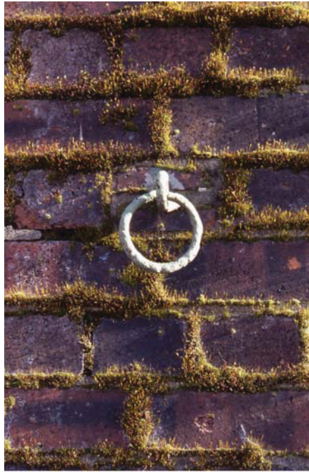
Plate 23 Detail of original metal ring on west elevation of Building 4, Stables, looking east
