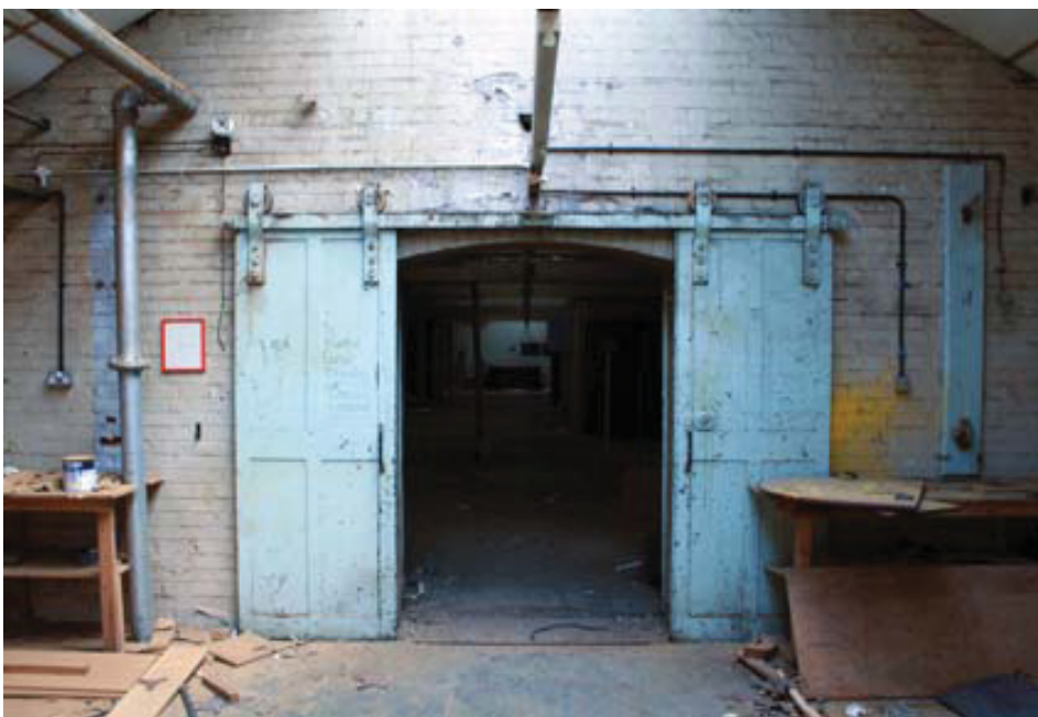
Plate 8 Internal view of Building 1, Starch Department, third floor detail of fire door, looking north
