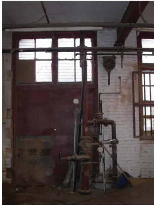
Plate 15 Internal view of Building 2, Lozenge Department, showing fire sprinkler machinery, looking south
