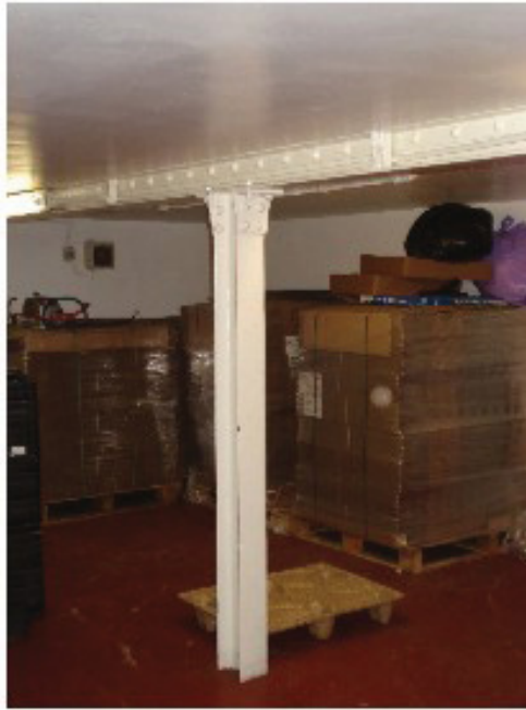
Plate 19 Internal view of Building 3, Peel Shed, detail of column in basement, looking east
