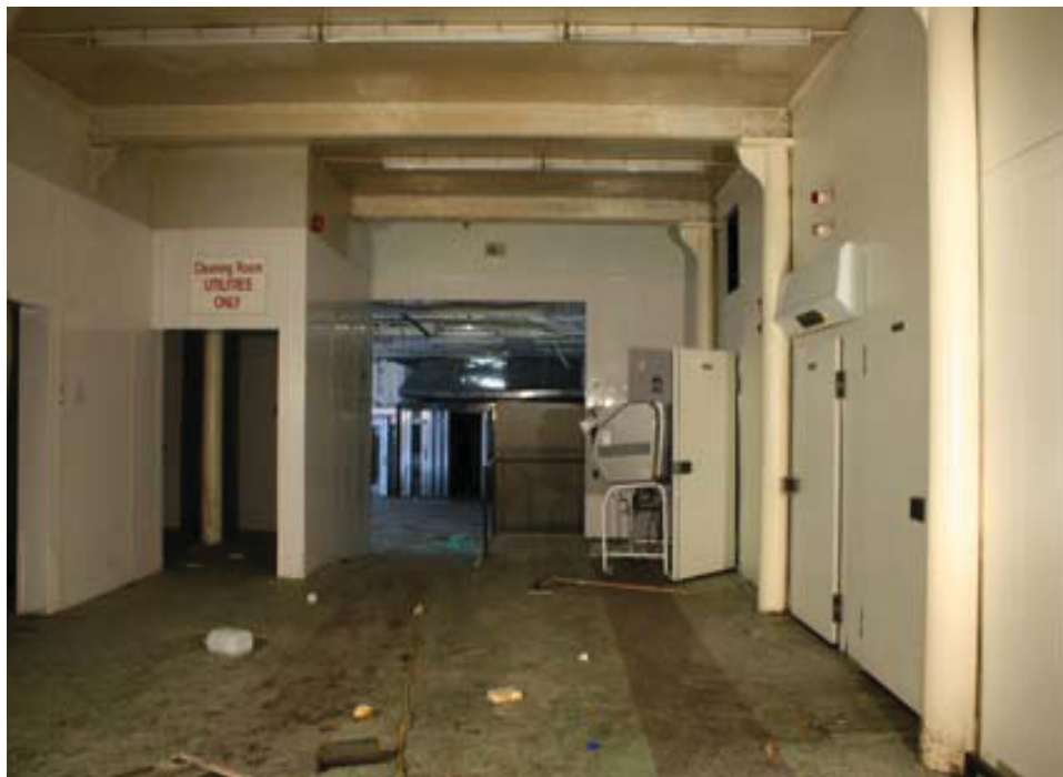
Plate 18 Internal view of Building 3, Peel Shed, detail of columns and layout of ground floor, looking west
