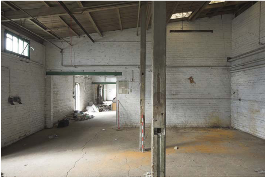
Plate 21 Internal view of Building 4, Stables, showing layout of one of the bays with timber supports, looking north
