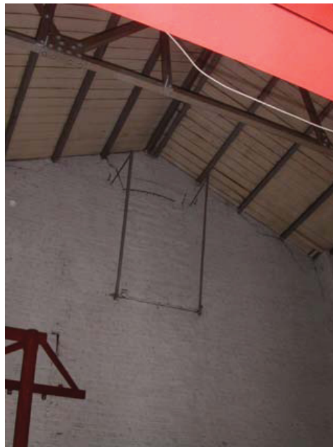
Plate 32 Detail of blocked opening near apex of roof inside Building 6, Engine House, looking east
