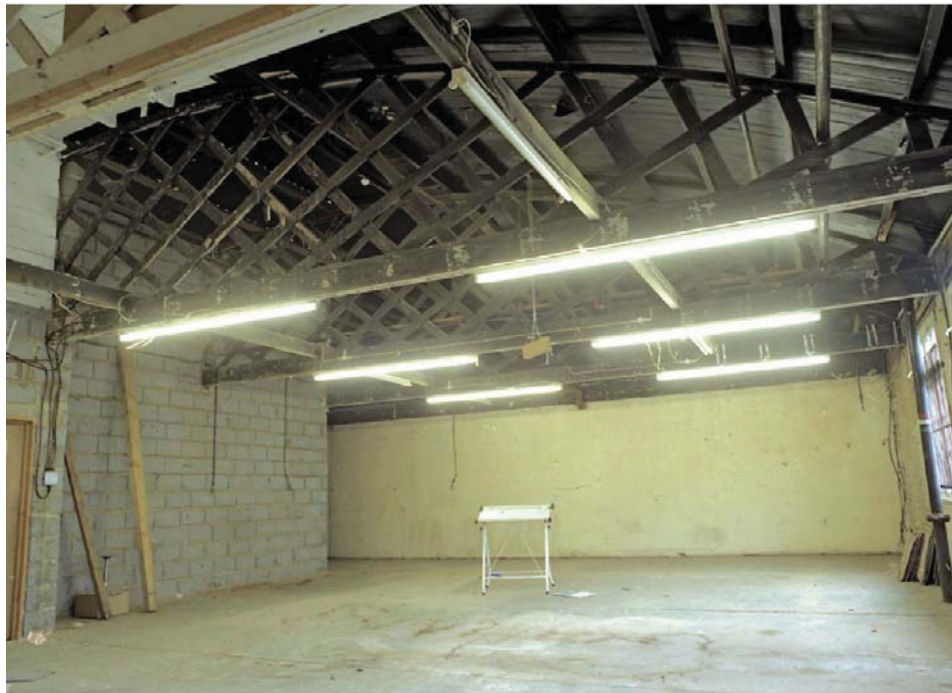
Plate 14 Internal view of Building 2, Lozenge Department, showing Belfast truss on the first floor, east end, looking west
