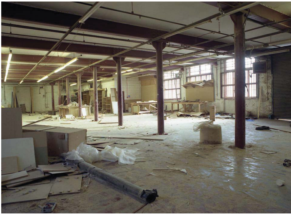
Plate 13 Internal view of Building 2, Lozenge Department, showing general layout and columns on the ground floor, looking south-east
