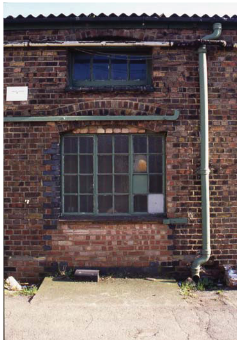
Plate 22 Detail of original doorway on west elevation of Building 4, Stables, looking east
