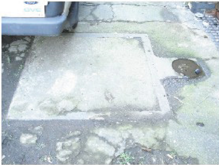
Plate 33 View of weigh plate to the south of Building 3, Peel Shed, looking east
