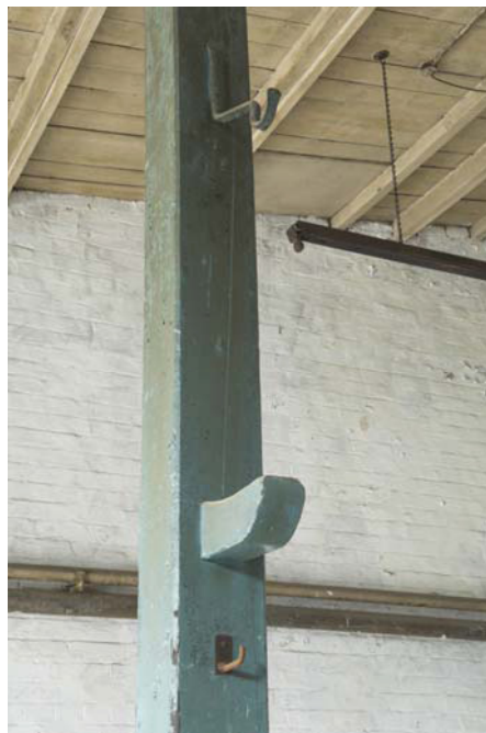
Plate 26 Detail of timber support showing original fitting in Building 4, Stables, looking north
