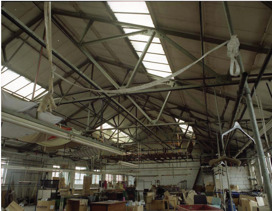
Plate 12 Internal view of Building 2, Lozenge Department, showing Fink trusses on second floor, west end, looking east
