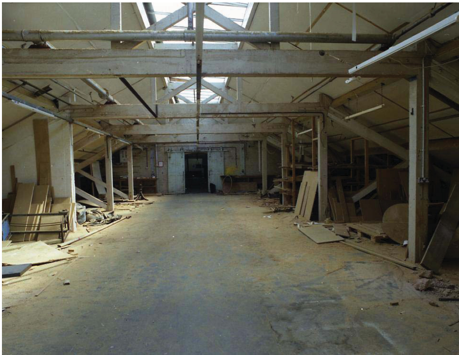
Plate 7 Internal view of Building 1, Starch Department, third floor showing timber truss with fire doors in the distance, looking north
