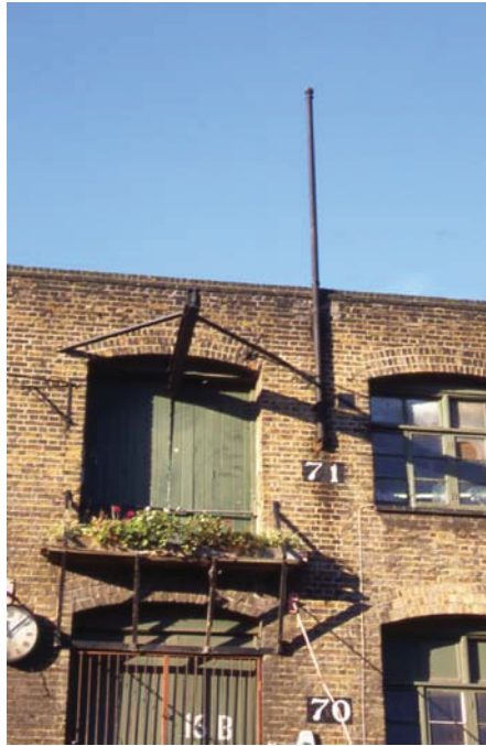
Plate 5 View of east elevation of Building 1, Starch Department, detail of loading door and flagpole, looking west
