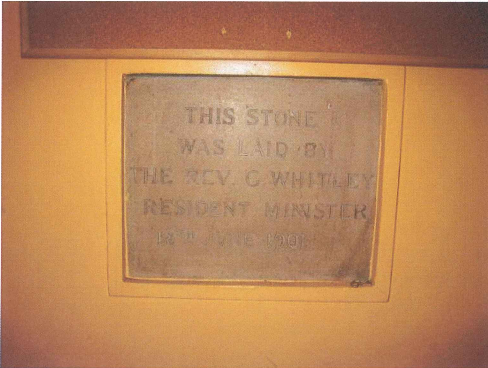
Plate 5: Foundation stone in the south wall of the main ground floor room of the 1902 entrance building
