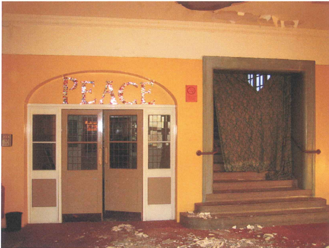
Plate 3: West wall of the main ground floor room of the 1902 entrance building
