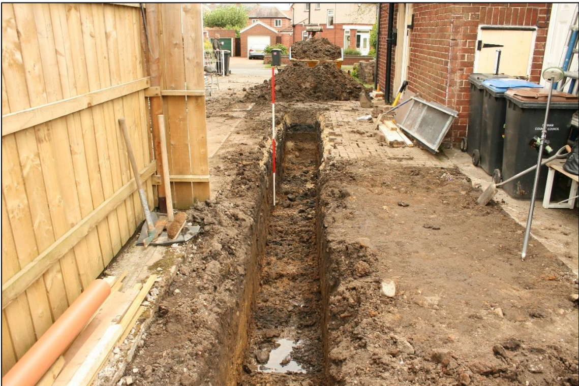
Plate 6- Overview of east-west orientated foundation trench, northern part of foundation trench, view east, 2m scale.
