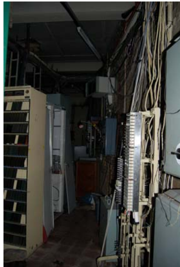
Plate 11: Relay room on ground floor
