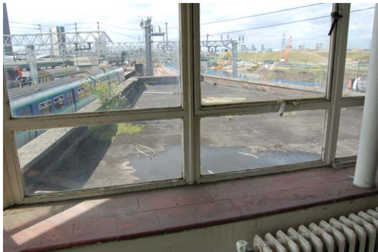
Plate 20: Metal window with ceramic tile sill in room F7 on first floor
