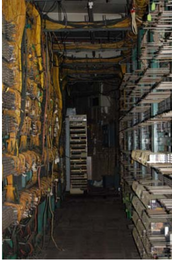
Plate 10: Relay room on ground floor
