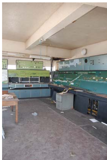
Plate 21: Signal control boards in room F7 on first floor
