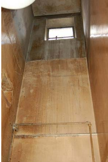
Plate 16: Small metal window at ceiling height in room F3 on first floor
