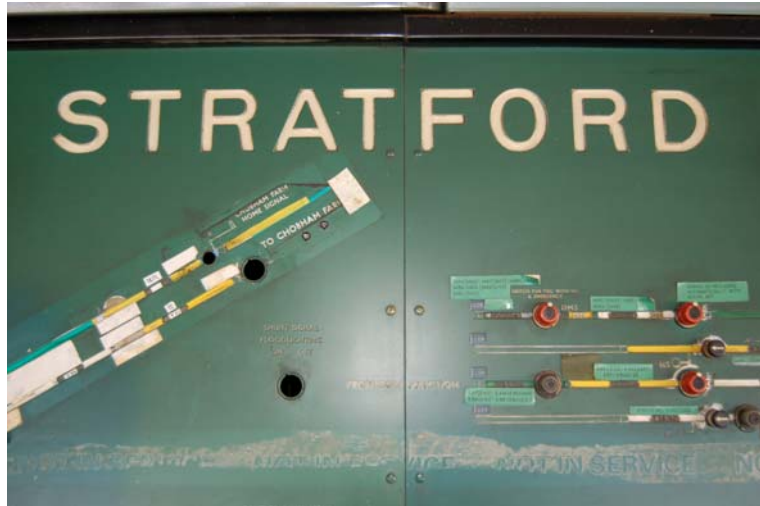
Plate 22: Signal control board in room F7 on first floor
