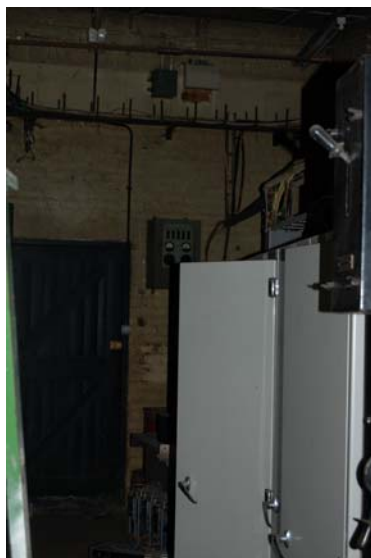
Plate 12: Relay room on ground floor
