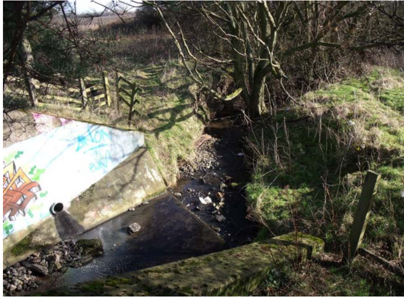
Plate 9. Exit to culvert of Seaton Burn tributary, east of the A189, looking north-east.
