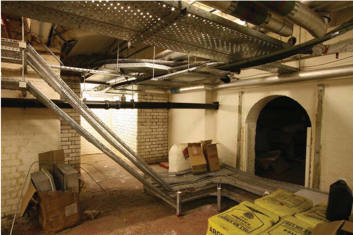
Plate 11: Bindery basement with blocked passage to the British Museum and archway to southern coal bunker on right.
