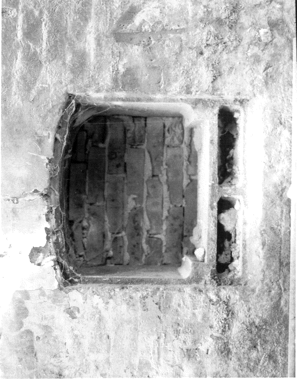
Figure 15 Bearing housing on the northern side of the western wall of the engine room
