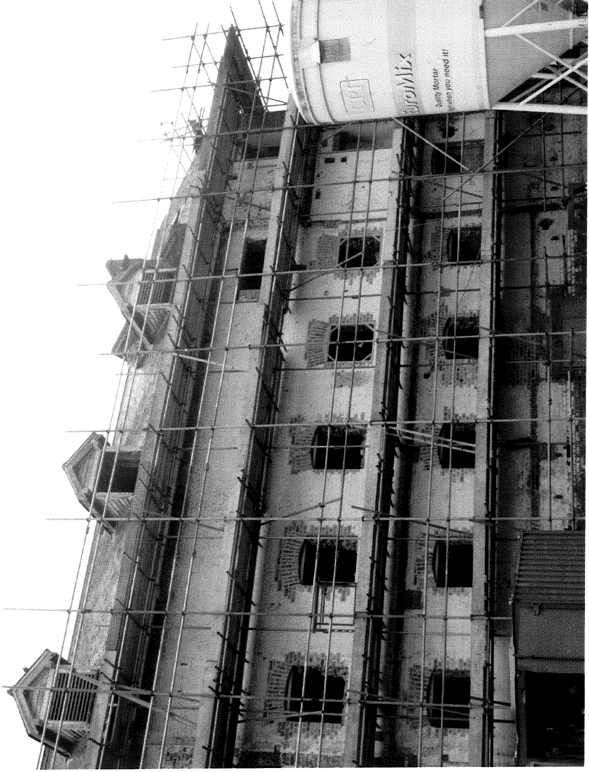
Figure 5 Photograph showing mill from southwest with the paintwork of the dismantled Atcos Building clearly visible
