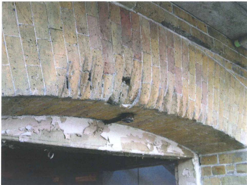
Figure 21 Rope/cable wear above the first floor loading doors on the north of the mill
