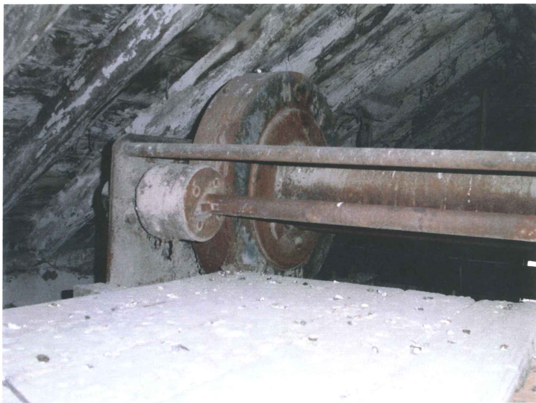
Figure 25 Cable drum and drive-roller of the hoist
