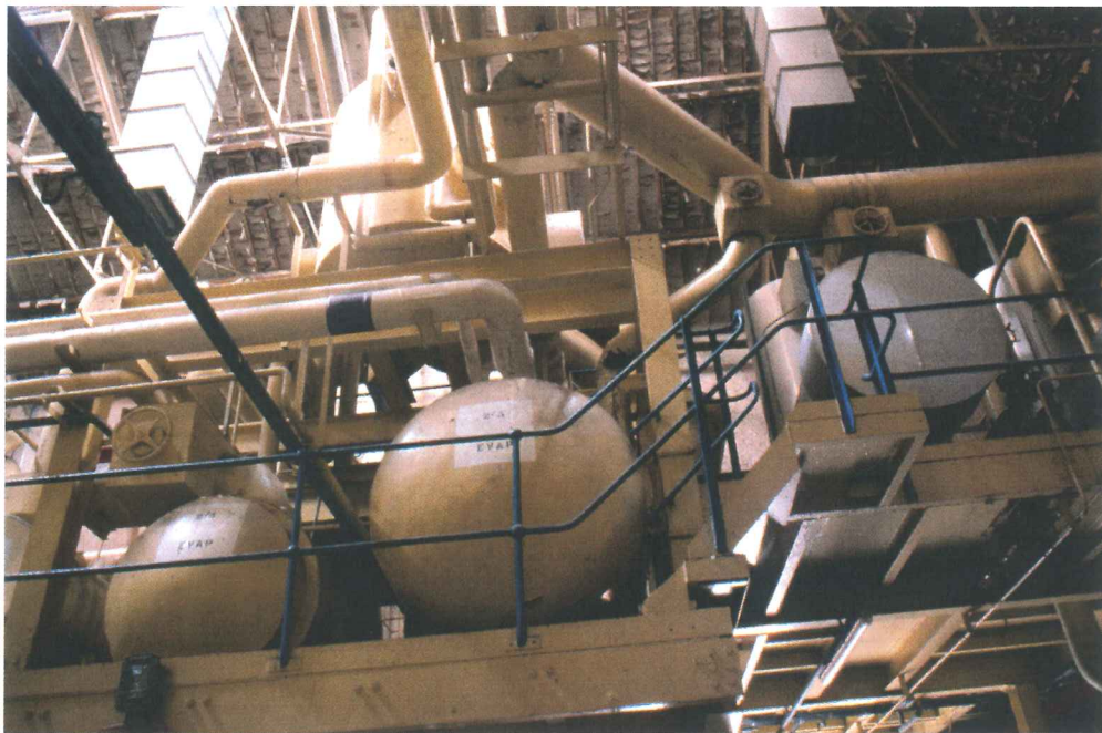
Plate 12: Tanks And Pipes In The Compressor Room
