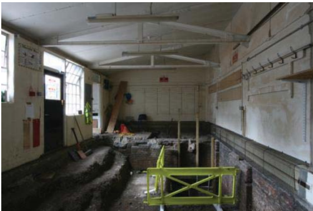
Plate 15. Trench 6, excavated workshop looking west. On the right are two blocked windows and in the centre the low wall is the original west wall of the basement, with a wide chimney breast and arched fireplace. The barriers in the foreground surround a deeper excavation exposing the foundations of the north and west basement walls.
