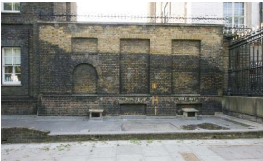
Plate 9. Trench 6, north facing elevation of carpenters' workshop north wall. The lowest section of red brick forms the basement of the original building, the infilled arched doorway relates to the porters lodge behind and the upper yellow brick section is associated with the construction of the workshop.
