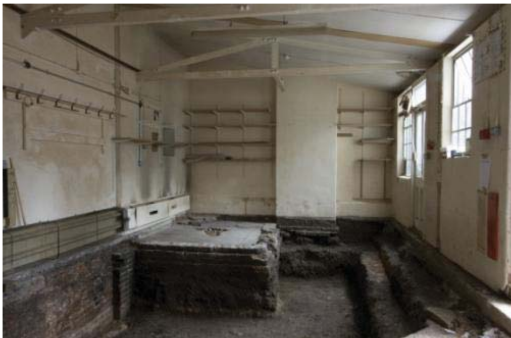
Plate 13. Trench 6, partially excavated workshop looking east with porters lodge floor left in situ. Noticeable on the left is an infilled basement window.
