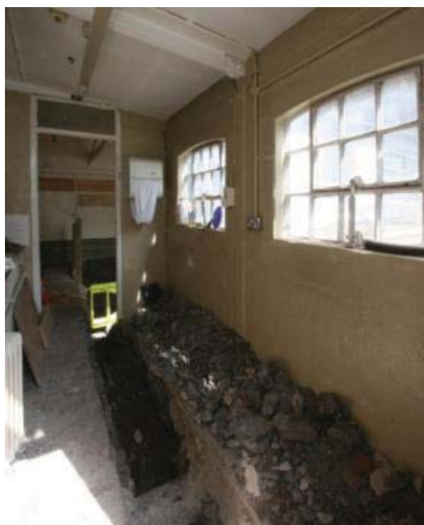
Plate 16. Trench 6, workshop kitchen looking north. In the foreground is a trench exposing the west basement wall.
