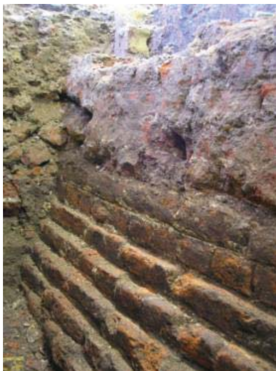
Plate 2. Trench 3, south facing elevation of Montagu House boundary wall, showing rebuild of upper section.
