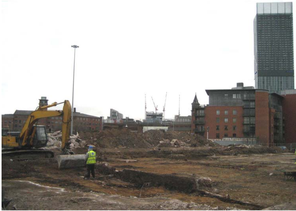
Plate 1. Machine excavation February 2008, north-western part of excavation area, looking north (Beetham Tower in rearground, right).
