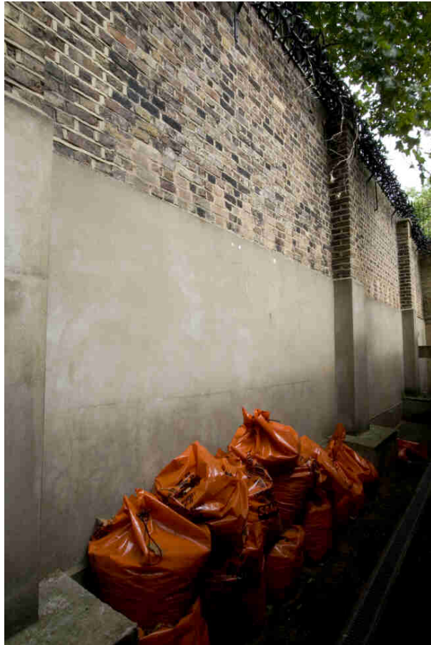
Plate 7 Line of infilled holes in south elevation of the boundary wall
