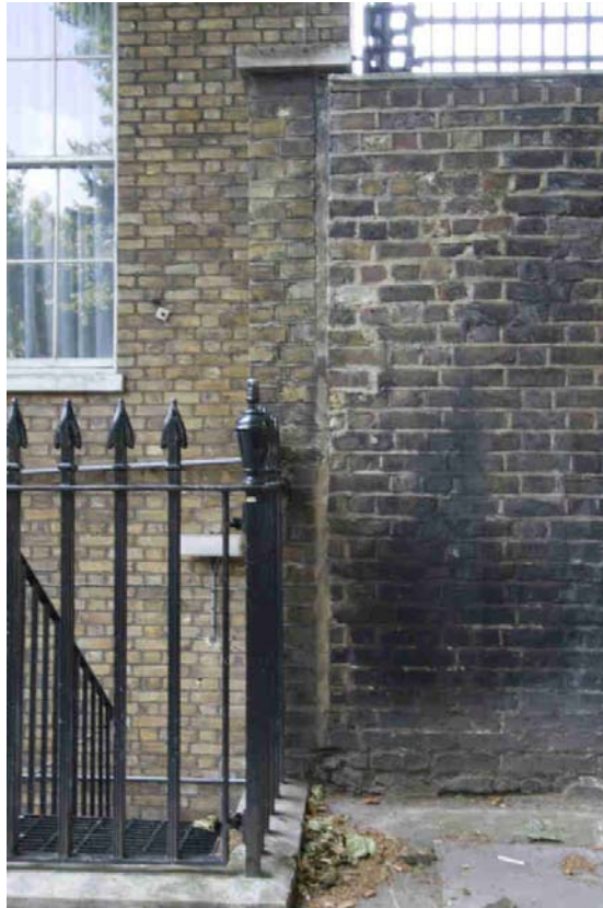
Plate 3 Straight joint at the east end of the boundary wall (view from the north)
