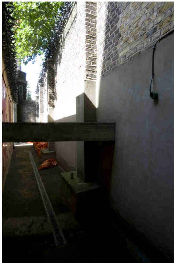
Plate 6 Concrete beam between the boundary wall and the substation (view from the east)
