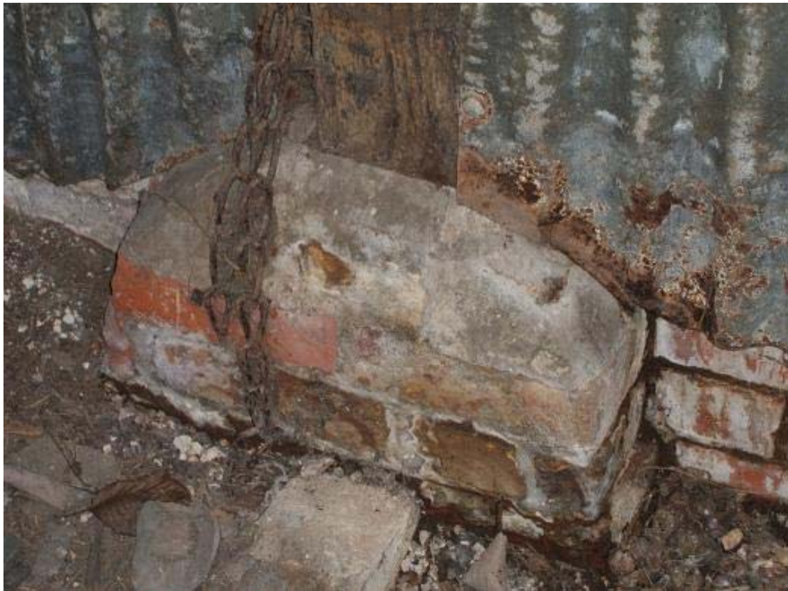
Plate 8: Brick pad supporting vertical timber post covered with cement viewed from the north-east (RG)
