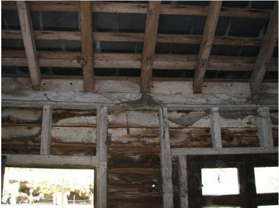
Plate 13: Rafters, wall plate and vertical stud work in the south-east elevation (RG)
