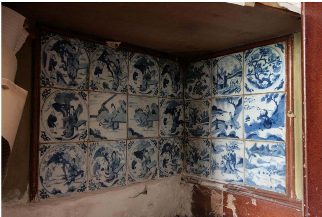
Plate 11 Second Floor, Tiles in cupboard in north-west corner of Mrs Soane's Morning Room (PCA)
