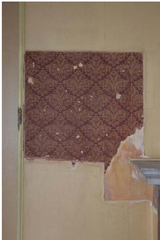
Plate 14 Second Floor Sir John Soane's Bedroom Opening 13 RmS/2-OU1 on east wall (PCA)
