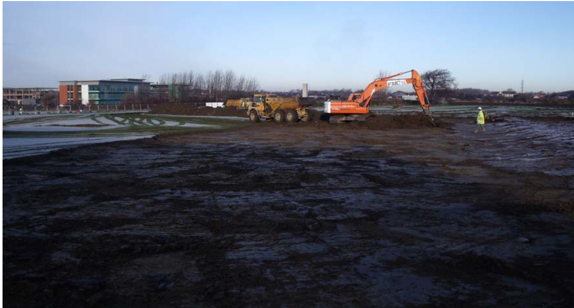
Figure 3. View of topsoil stripping, east end of new build footprint in Area 2, January 2009, looking south-west.
