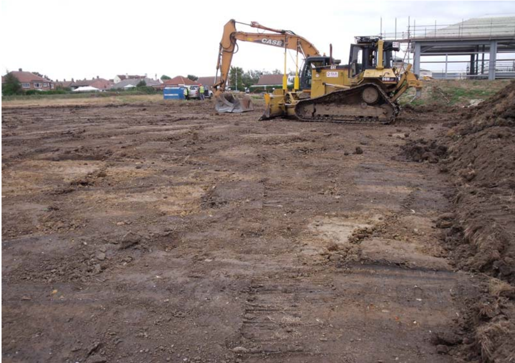
Figure 4. View of stripped area, west end of football pitch in Area 2, September 2009, looking south
