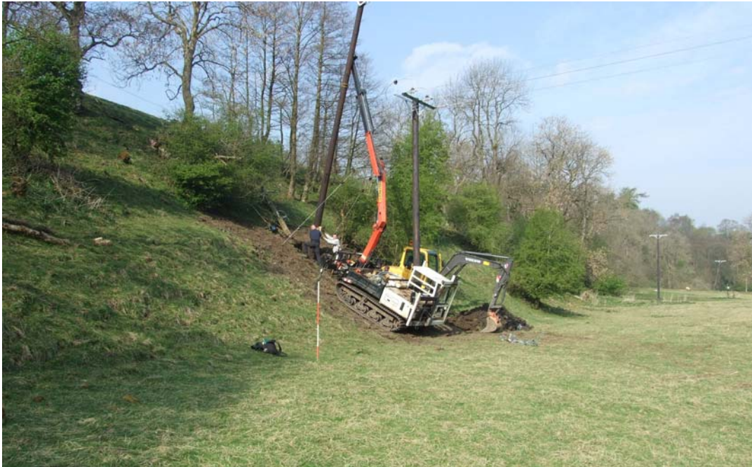
Figure 5: South end of Area 2, working shot at Pole 55, looking west (scale 2m).
