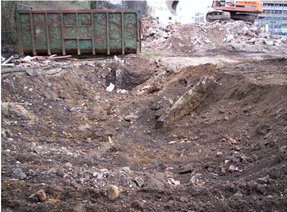
Image 7: Area of Truncation from Previous Construction, West End of Site, Facing East
