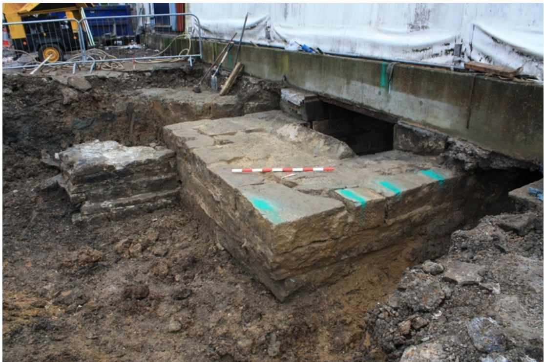
Plate 4. OP102. Chute/buttress structure [68] at an early stage of dismantling. The stone foundation [33] is to the top left. Scale 1.0m, looking south-east.
