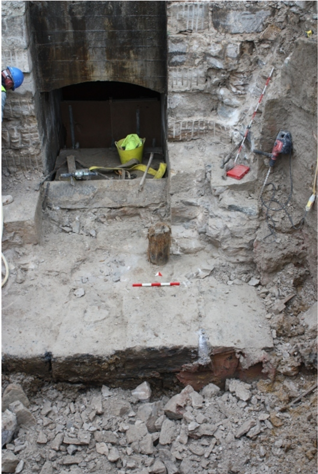
Plate 10. OP104. Chute/buttress [74] with timber post [82] at a later stage of dismantling. Scale 0.5m, looking north.
