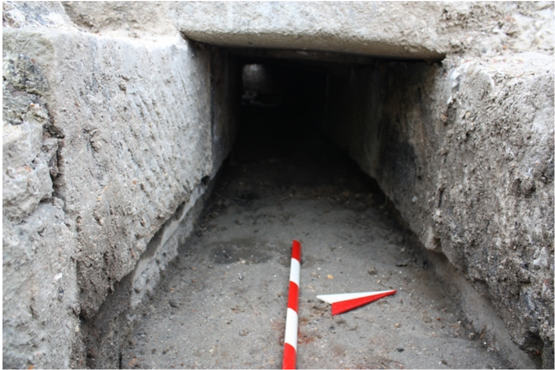
Plate 17. Area B. Detail of culvert [35], part of structure [37]. Scale 0.5m, looking west.
