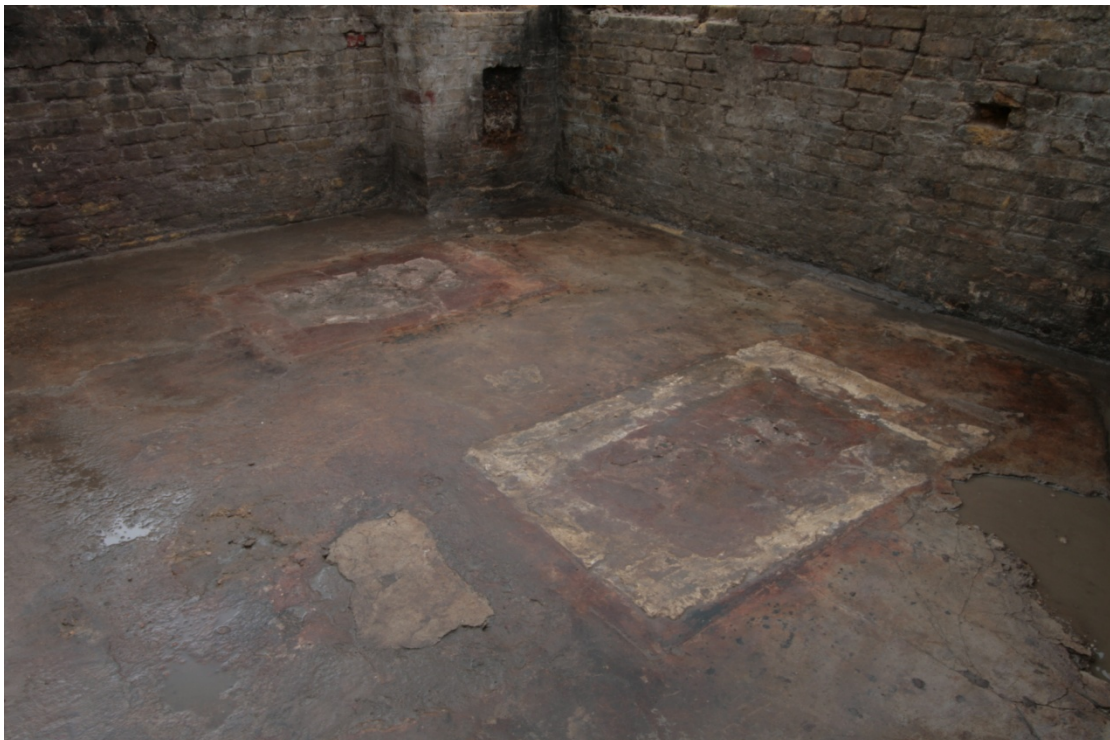
PLATE 4: MACHINE PADS WITHIN PUMP ROOM OF POOL-HOUSE, LOOKING SOUTH-WEST
