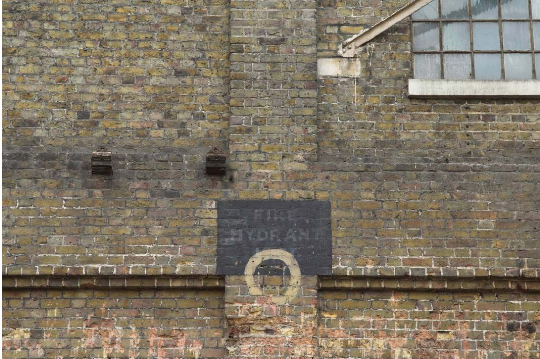
Plate 13: Fire Hydrant sign between Bays 5 and 6 in the west elevation (see Figure 14 and Plate 1 for location) of the MGS
