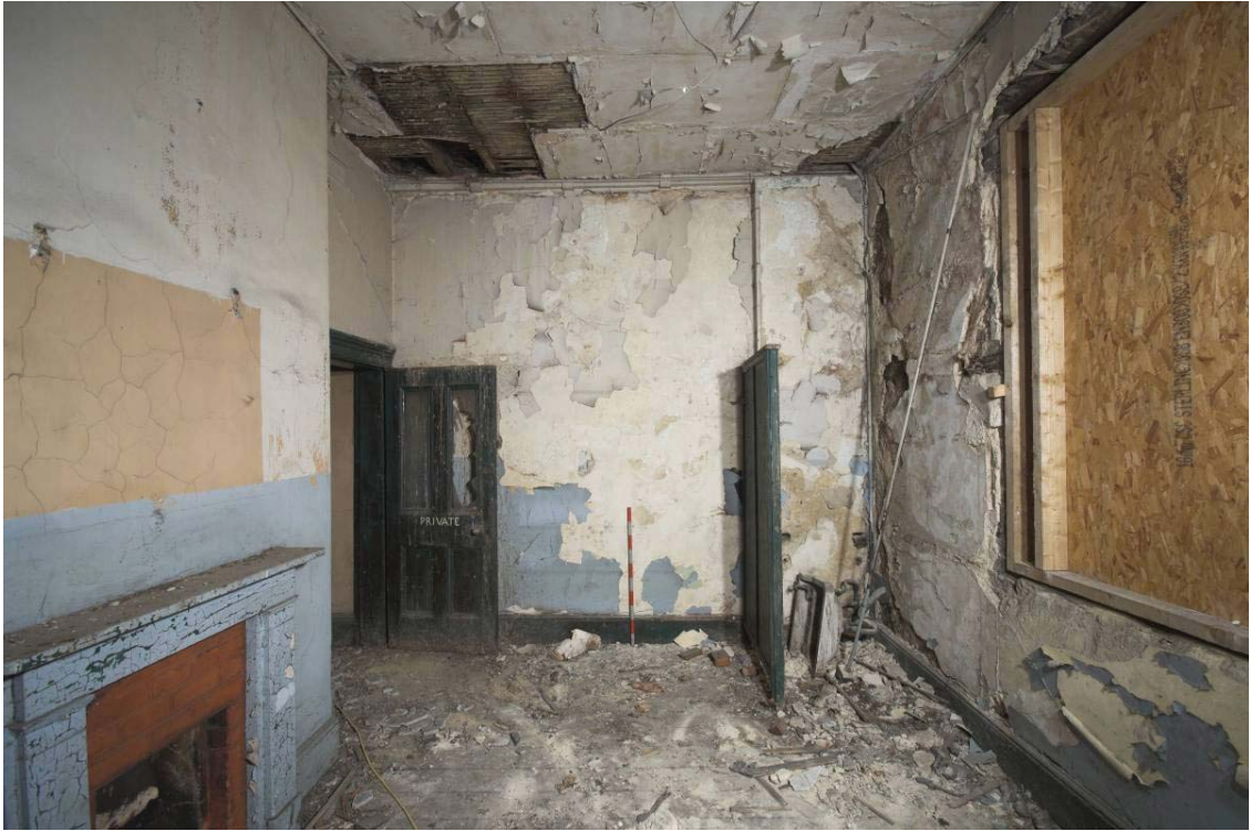
Plate 61: West, north and east wall of first floor MGS Office MGSOF6, view from the south
