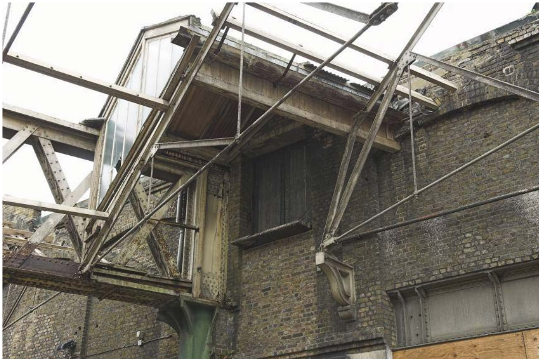
Plate 6: Loading doors and West Handyside Canopy truss with ornate iron bracket on stone corbel in Bay 20 of the west elevation of the MGS
