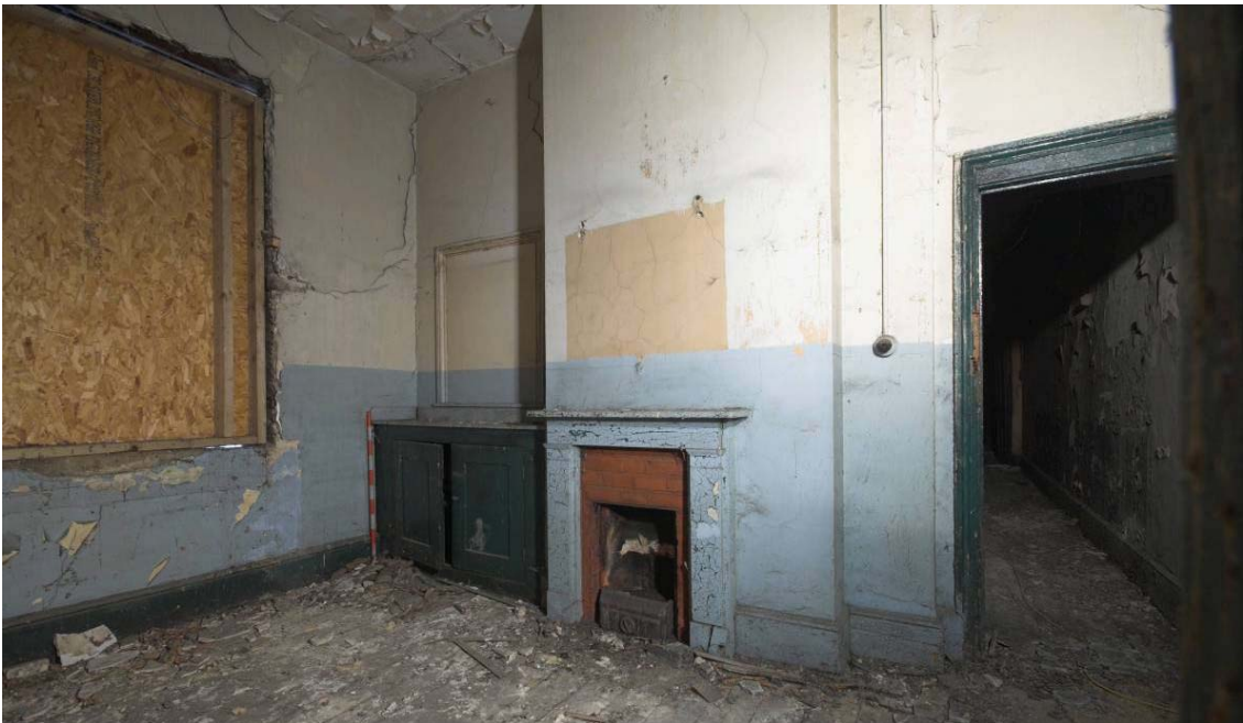
Plate 62: South and west wall of first floor MGS Office MGSOF6, view from the north-west
