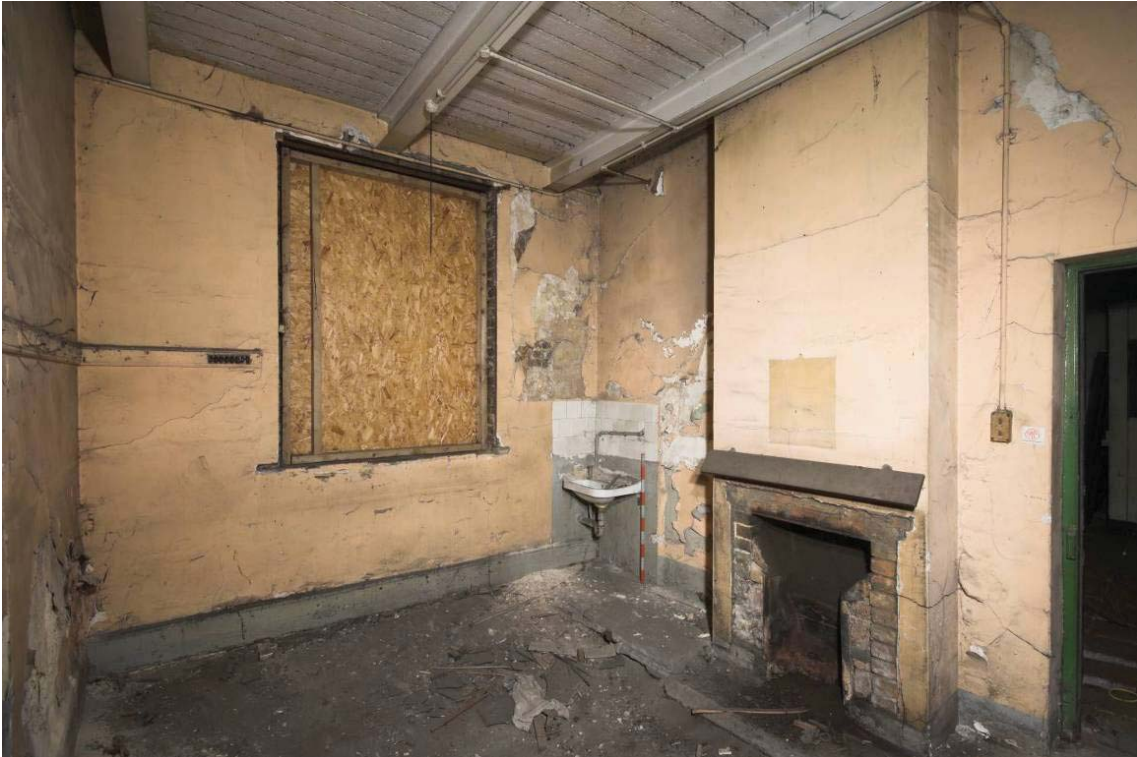
Plate 57: East, south and west wall of ground floor MGS Office MGSOG8, view from the north-east
