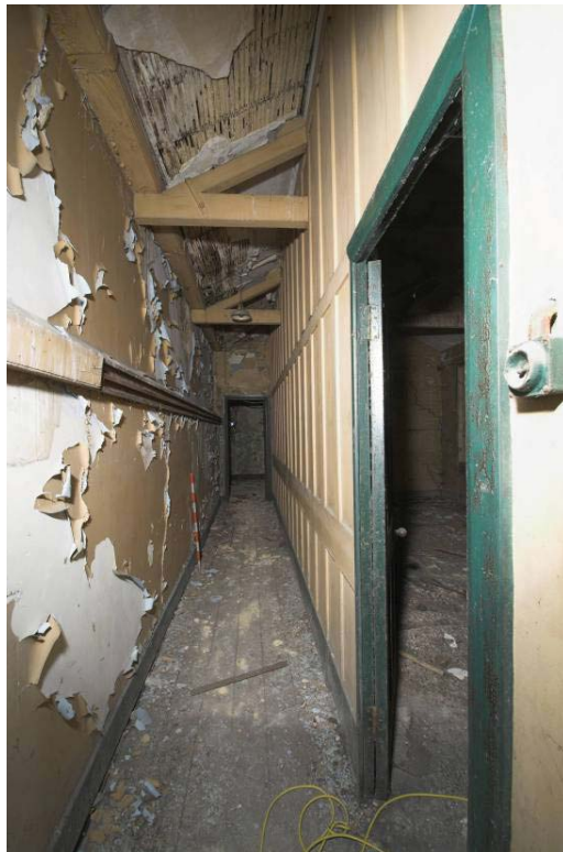
Plate 70: North, east and south wall of MGS Office Corridor MGSOS3, view from the west
