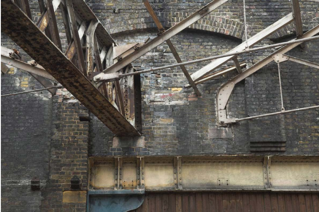
Plate 11: West Handyside Canopy girder and roof truss inserted above Loading Bay W1 in Bay 3 of the west elevation of the MGS
