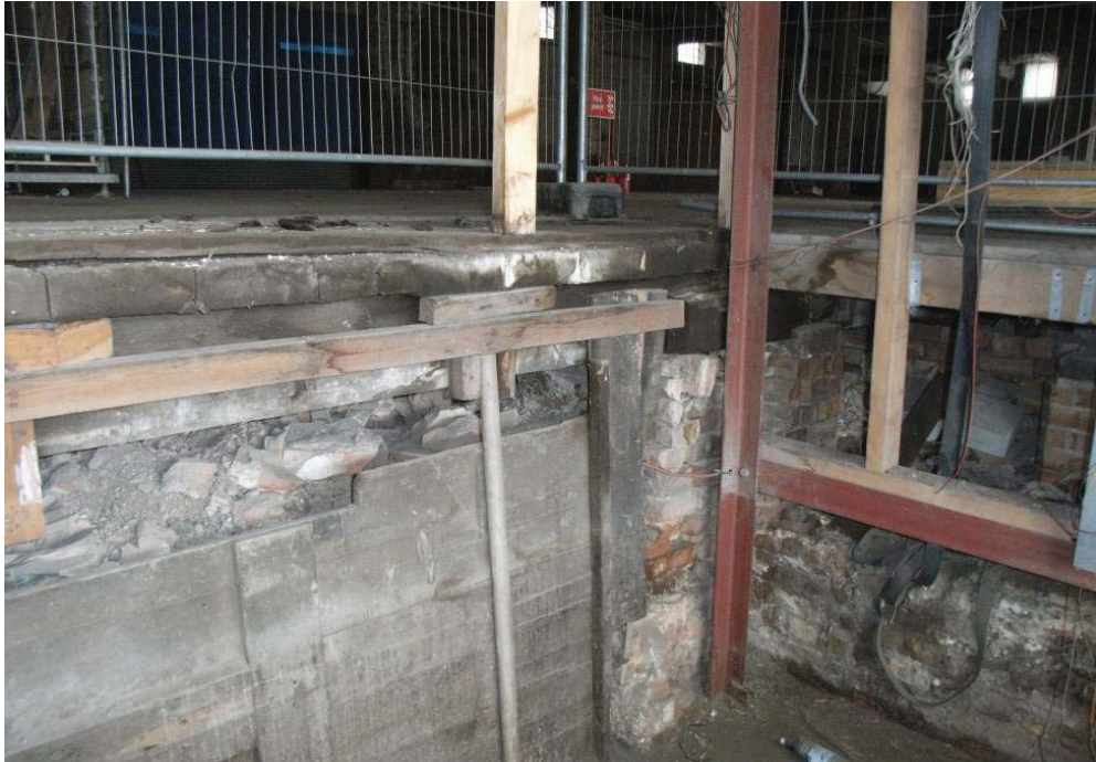
Plate 43a: North-west corner of lift shaft in Bay 11 (east side) of the MGS showing construction of the platform
