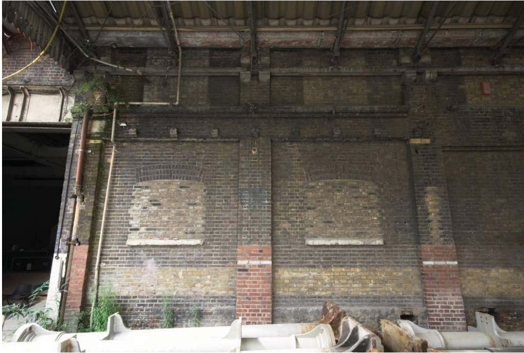
Plate 21: Bays 19 and 20 in the east elevation of the MGS showing lower flange of cast iron beam spanning 1858 opening (now infilled)
