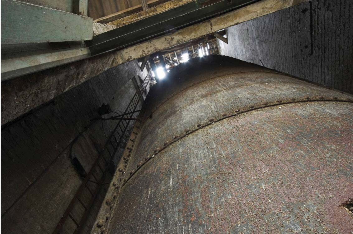
Plate 47: Hydraulic accumulator mechanism within the accumulator tower; south wall with ladder (left); north wall to right
