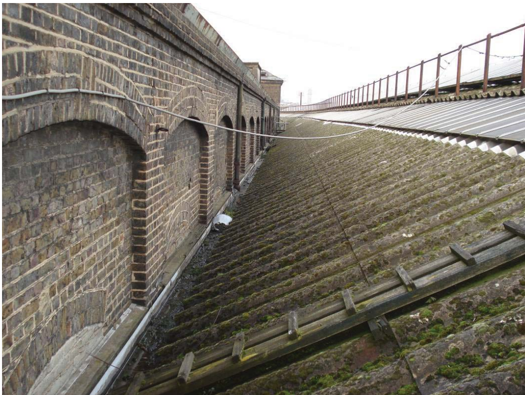
Plate 22: Upper part of the east elevation of the MGS (Bays 7 to 20; left) and East Handyside Canopy (right), view from the south
