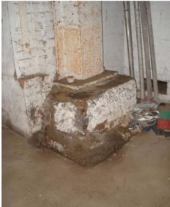
Plate 40: The base of a hollow cast iron side column in Pump House MGSG2 of the MGS, view from the north-west
