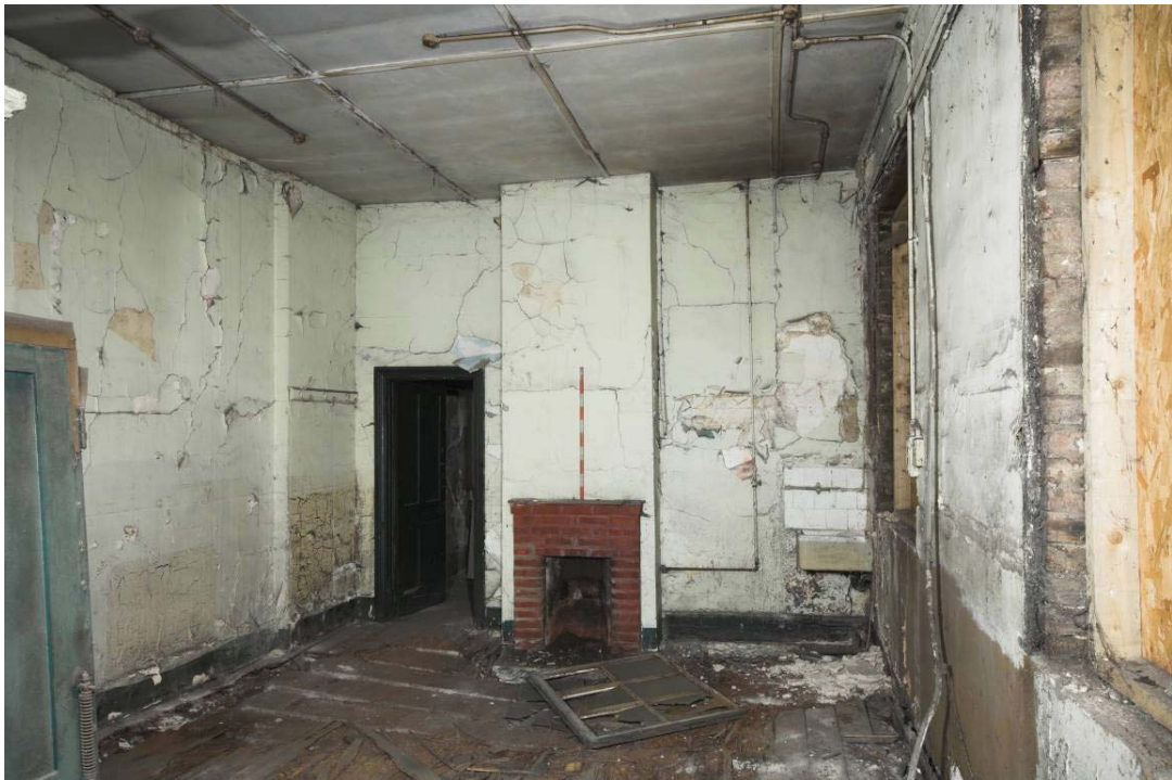
Plate 54: North, east and south wall of ground floor MGS Office MGSOG7, view from the west
