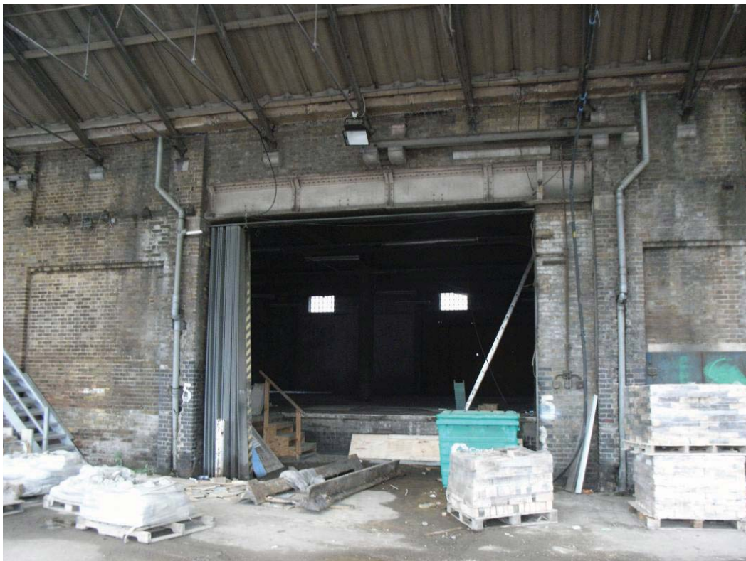
Plate 26: Loading Bay Opening E1 in the east elevation (Bays 2 to 5) of the MGS
