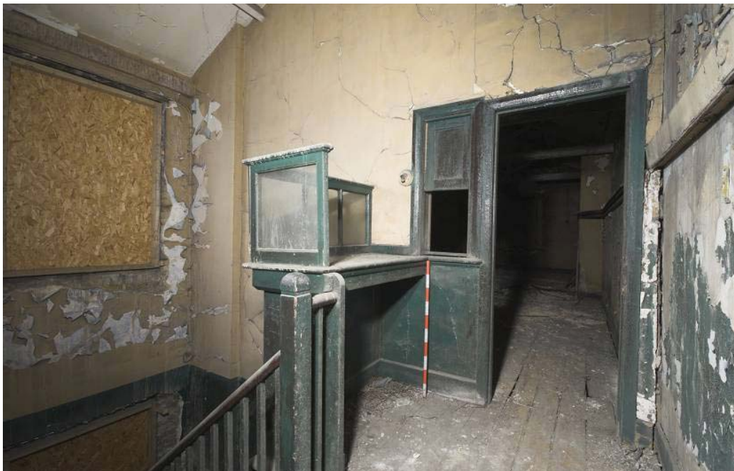
Plate 64: South, west and north wall of MGS Office MGSOS2 showing desk on second floor landing, view from the east
