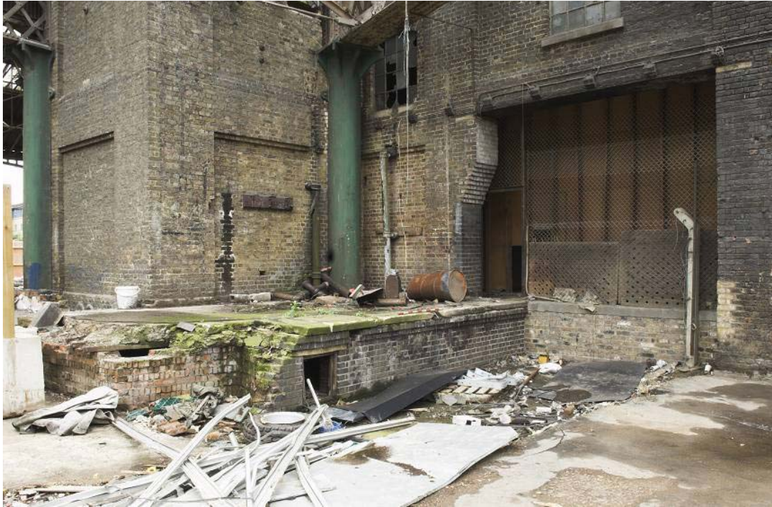
Plate 17: North and west elevation of the accumulator tower (left) and east end of the north elevation of the MGS (right) showing canopy columns, platform and east train entrance
