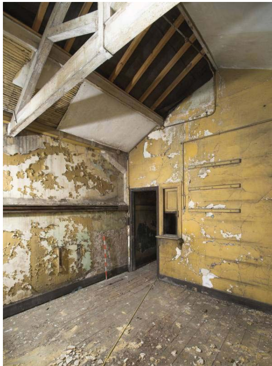
Plate 68: North and east wall of MGS Office MGSOS1, view from the south-west
