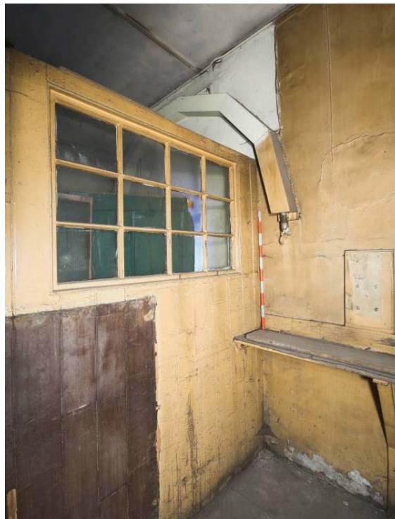
Plate 56: South and west wall of ground floor MGS Offices 'telephone' cubicle MGSOG9, view from the north-east
