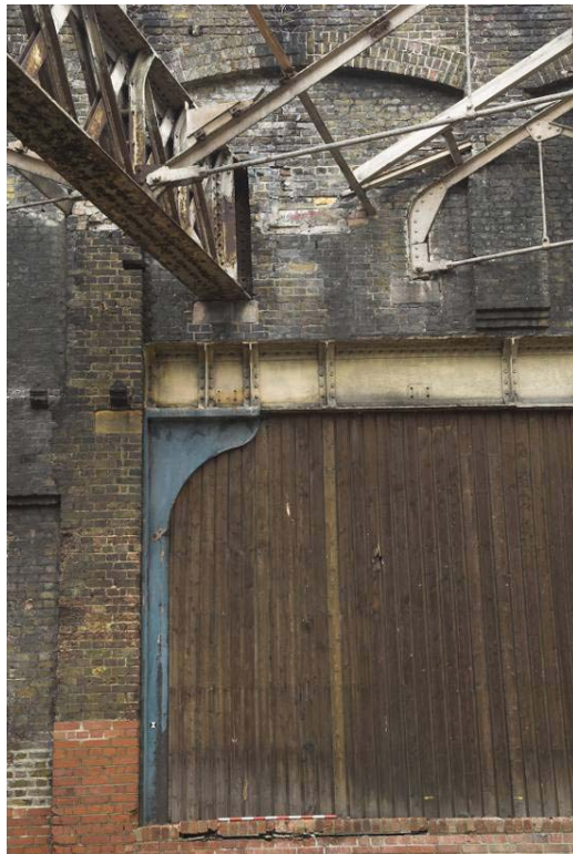
Plate 10: West Handyside Canopy girder and roof truss inserted above Loading Bay W1 in Bay 3 of the west elevation of the MGS
