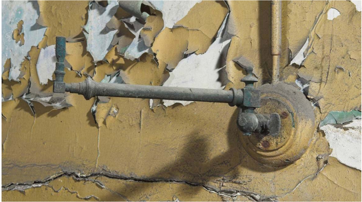
Plate 65: Gas light fitting on the south wall of MGS Office MGSOS1, view from the north-east
