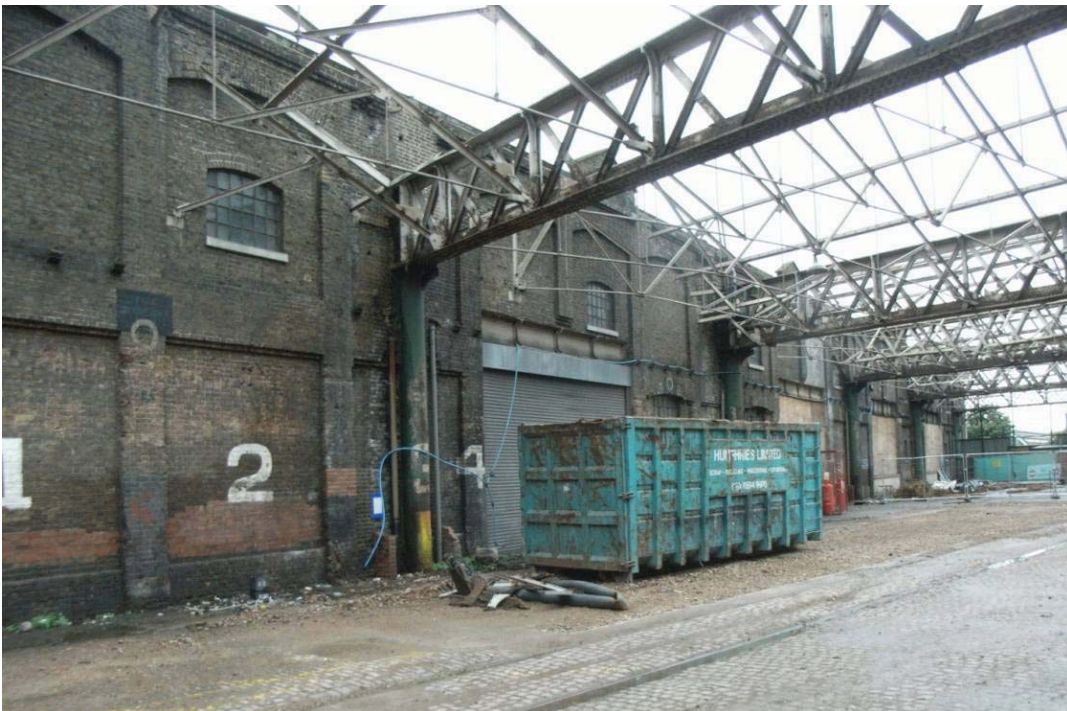
Plate 2: View towards the southern end of the west elevation (Bays 5 to 24) of the MGS
