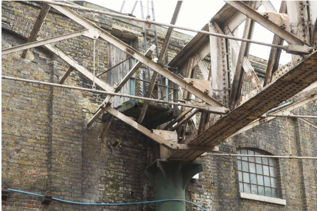
Plate 5: Loading door and roof access in Bay 11 of the west elevation of the MGS
