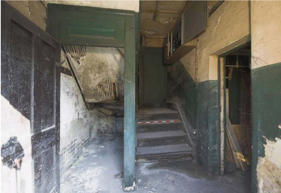
Plate 53: West, north and east wall of ground floor MGS Office entrance hall MGSOG6 with former doorway to the MGS in the north wall, view from the south
