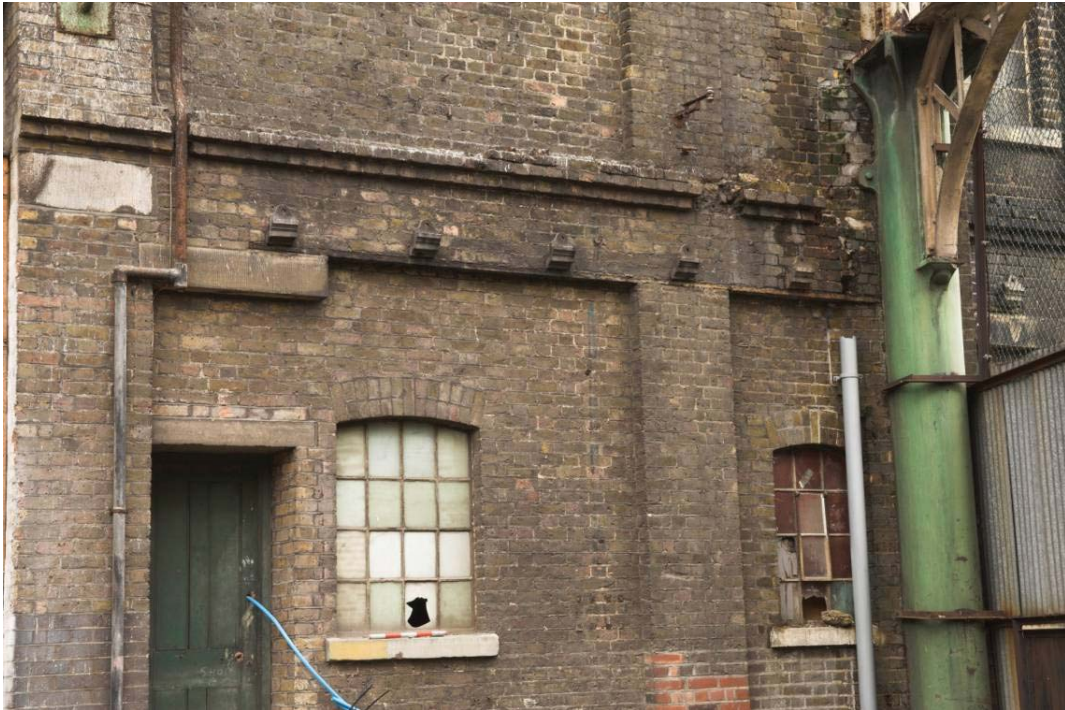
Plate 4: Bays 23 and 24 in the west elevation of the MGS showing lower flange of cast iron beam spanning 1858 opening (now infilled)
