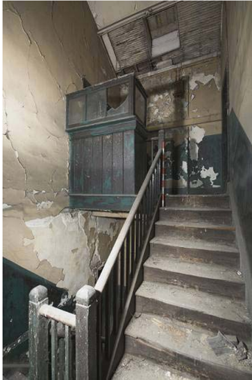
Plate 63: West, north and east wall of MGS Office Stairwell MGSOS2 showing second floor landing and desk, view from the south
