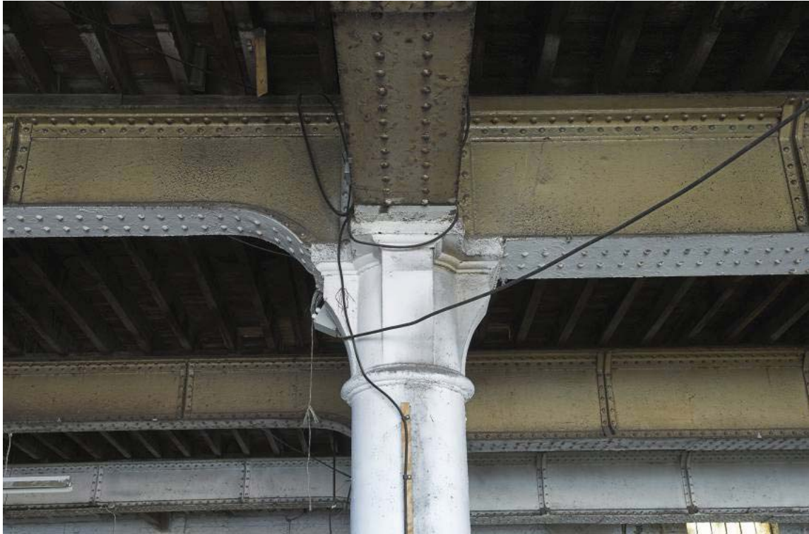
Plate 37: Column capital and ceiling girders supporting the first floor of the MGS
