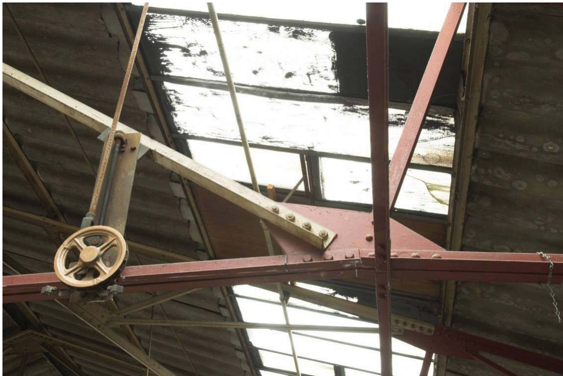
Plate 32: Pulley wheel system on roof truss which opens panels in the skylight of the MGS
