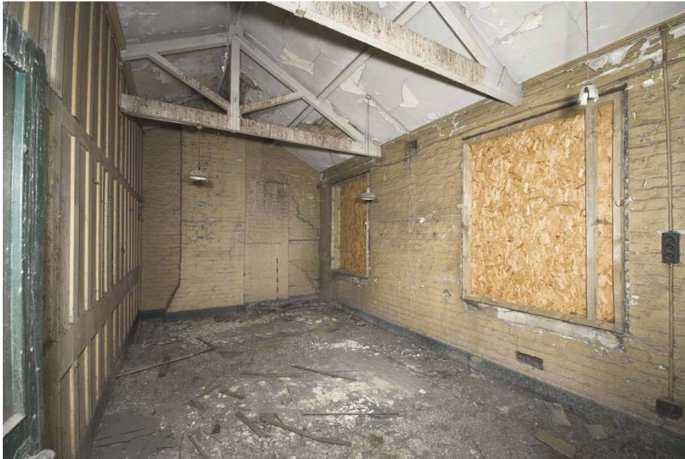
Plate 69: North, east and south wall of MGS Office MSGOS4, view from the west
