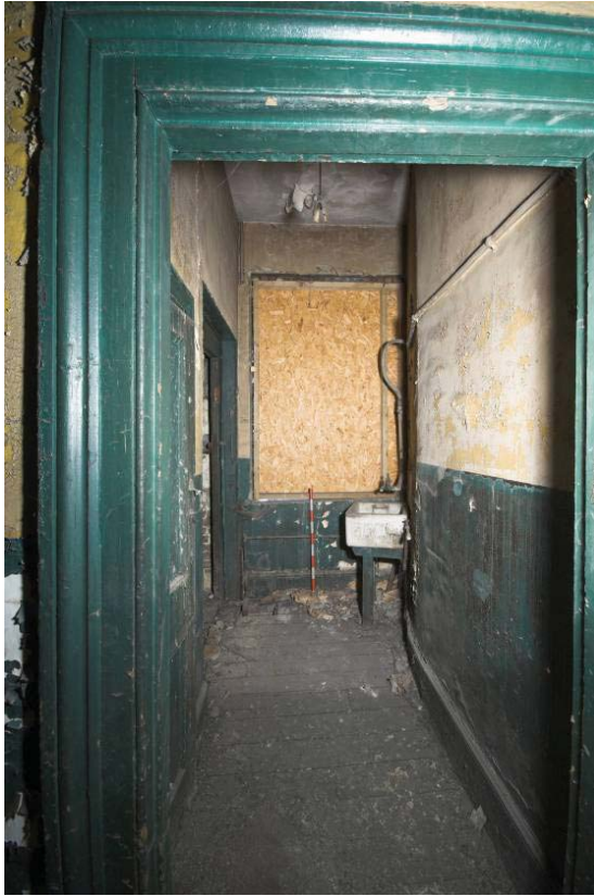
Plate 59: East, south, and west wall of first floor MGS Office MGSOF3, view from the north
