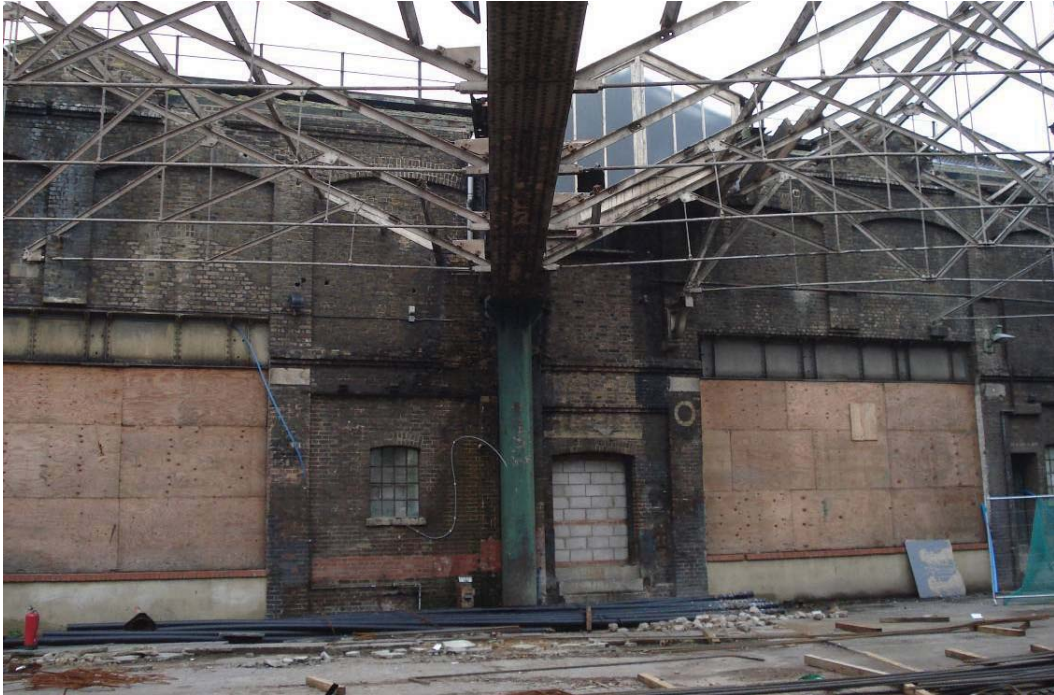
Plate 3: Loading Bays W4 and W5 in the west elevation (Bays 18 to 22) of the MGS
