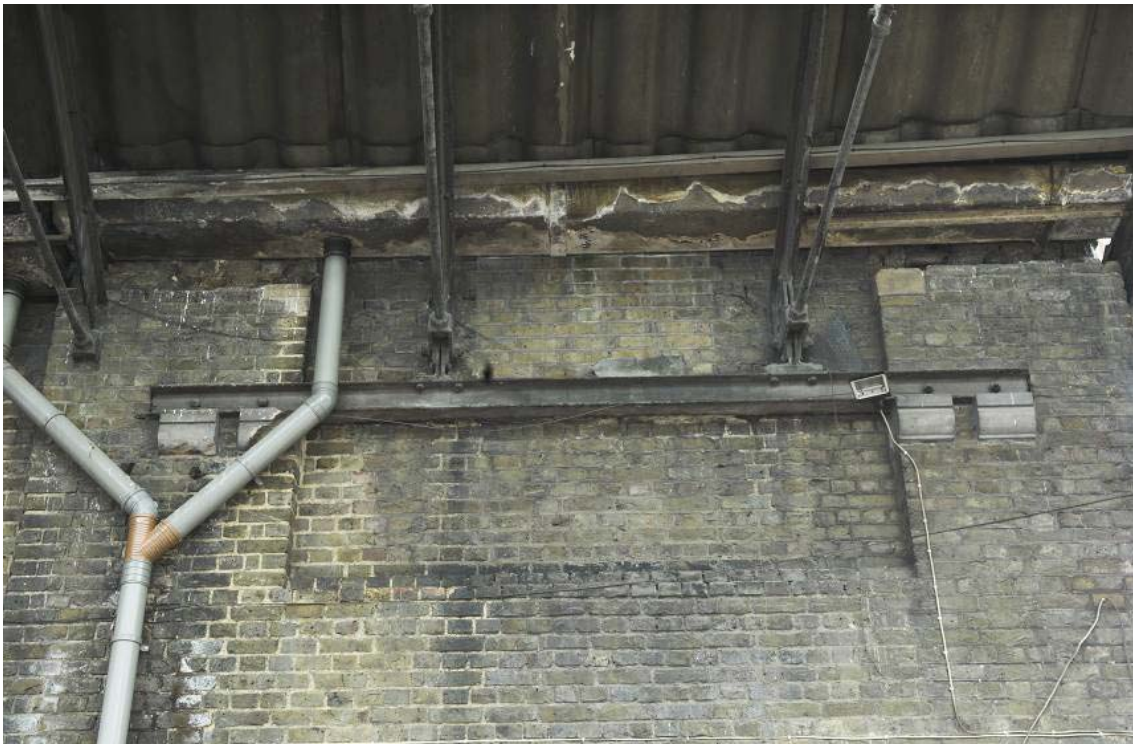
Plate 46: Blocked first floor window in the east elevation of the accumulator tower with girder across to support trusses for the East Handyside Canopy
