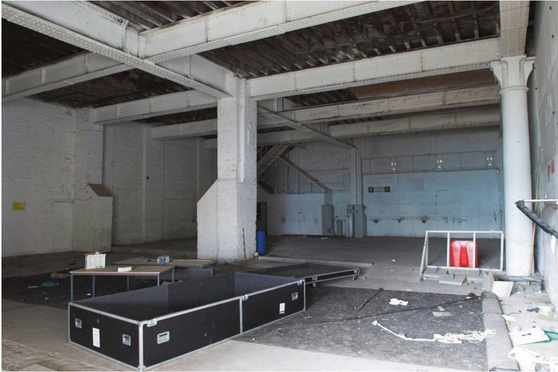
Plate 39: South end of the ground floor of the MGS, view from the north-east
