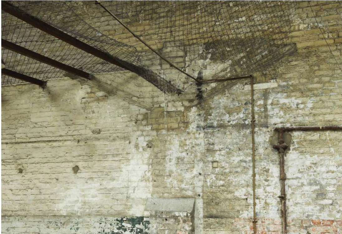
Plate 29: Valley of the former double gable roof visible in the brickwork of the south wall of the MGS
