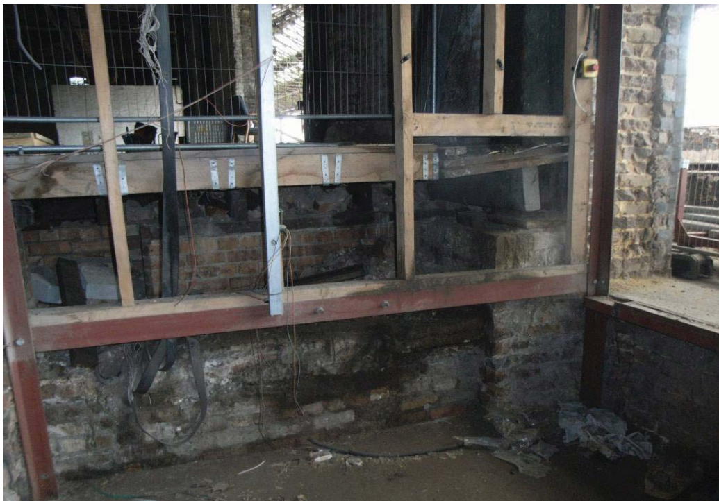
Plate 42: North side of the lift shaft in Bay 11 (east side) of the MGS showing construction of the platform
