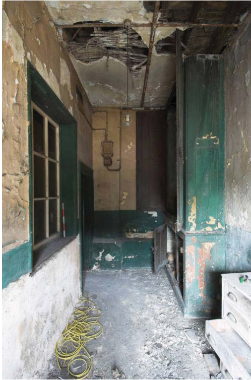
Plate 49: West, north and east wall of ground floor MGS Office Room MGSOG5, view from the south
