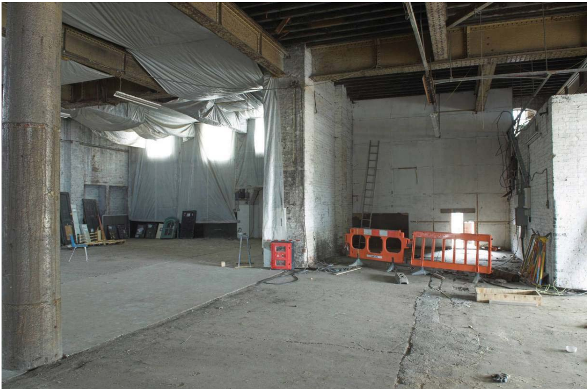
Plate 38: North end of the ground floor of the MGS, view from the south-east
