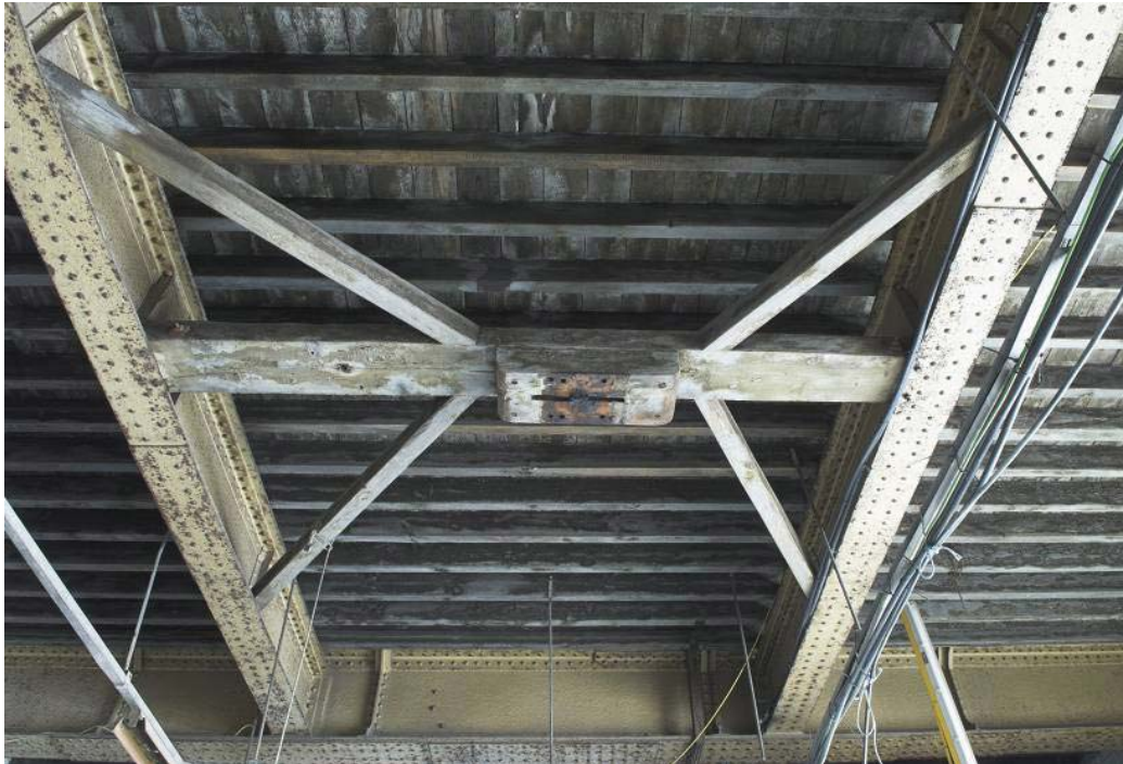
Plate 41: Ceiling-mounted fixing under the first floor of the MGS for a swivelling platform crane, view from the south
