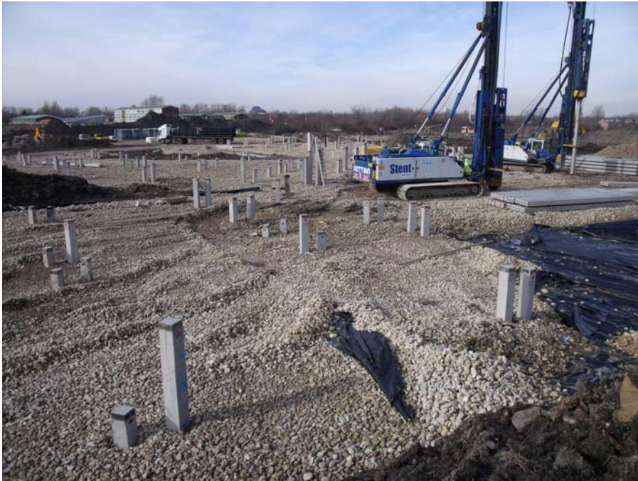
Figure 3. Overview of construction groundworks (3 March 2010), looking west across the main new build footprint
