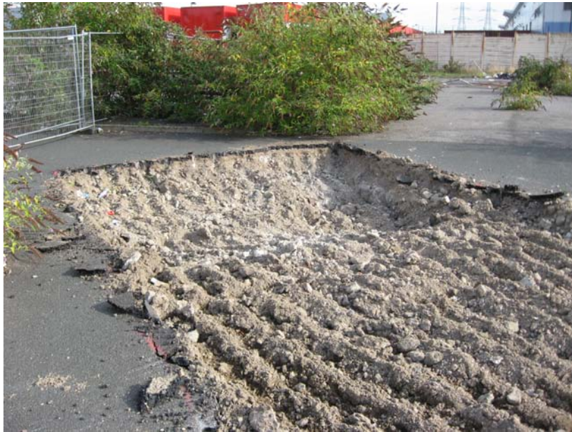
Plate 1: NW end of Trench 1 showing severe concrete intrusions
