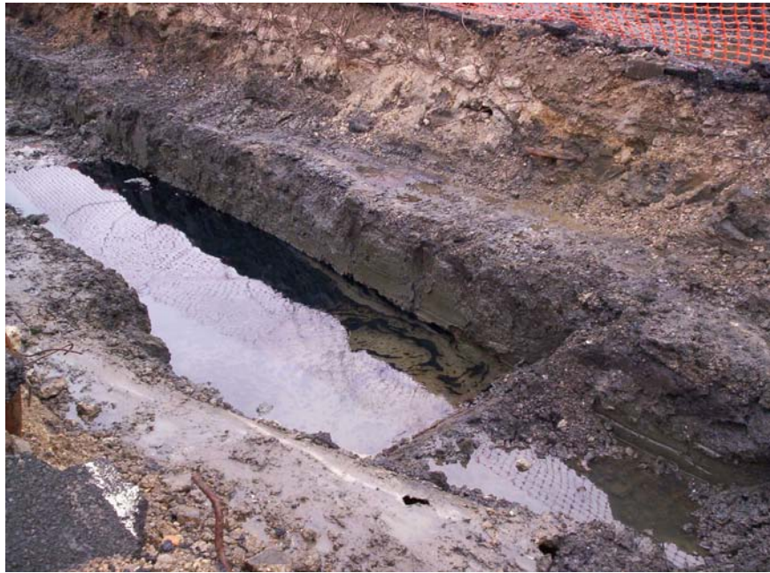
Plate 3: South-eastern end of Trench 3 showing oil contamination
