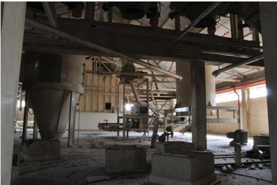
Machine bases on second floor in the Mill's eastern extensions (see Figure 13 for location), view to south-east
