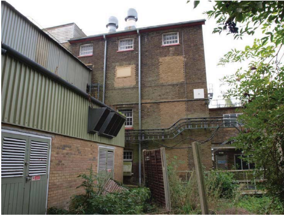
West end of Mill's north elevation (see Figure 2 for location). View to south-east.
