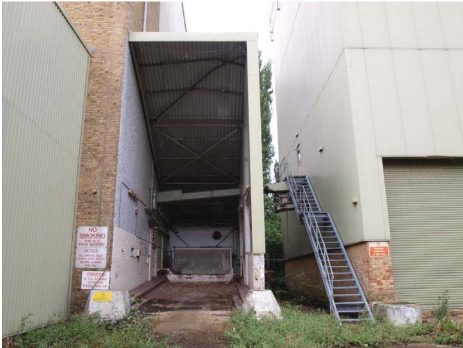
South loading bay, northern extension of the Mill (see Figure 2 for location), view to west.
