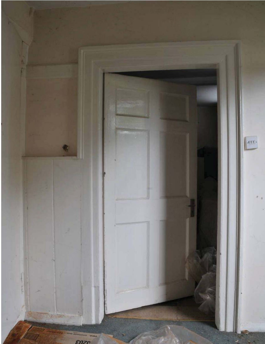
Original door and panelling, ground floor of Kingsmill Cottage (see Figure 24 for location). View to south.
