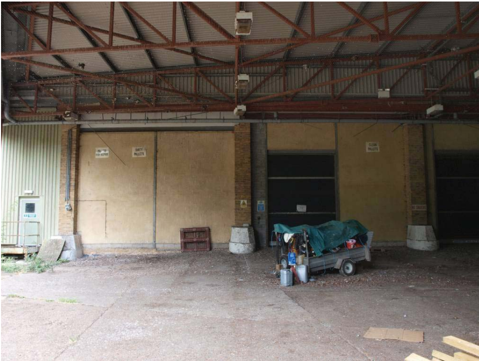
South elevation of loading bay in the northern extension of the Mill (see Figure 2 for location), view to south.
