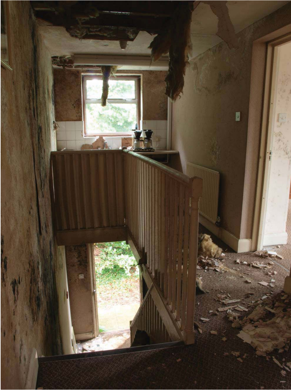
First floor landing, Mill House (see Figure 22 for location), view to south
