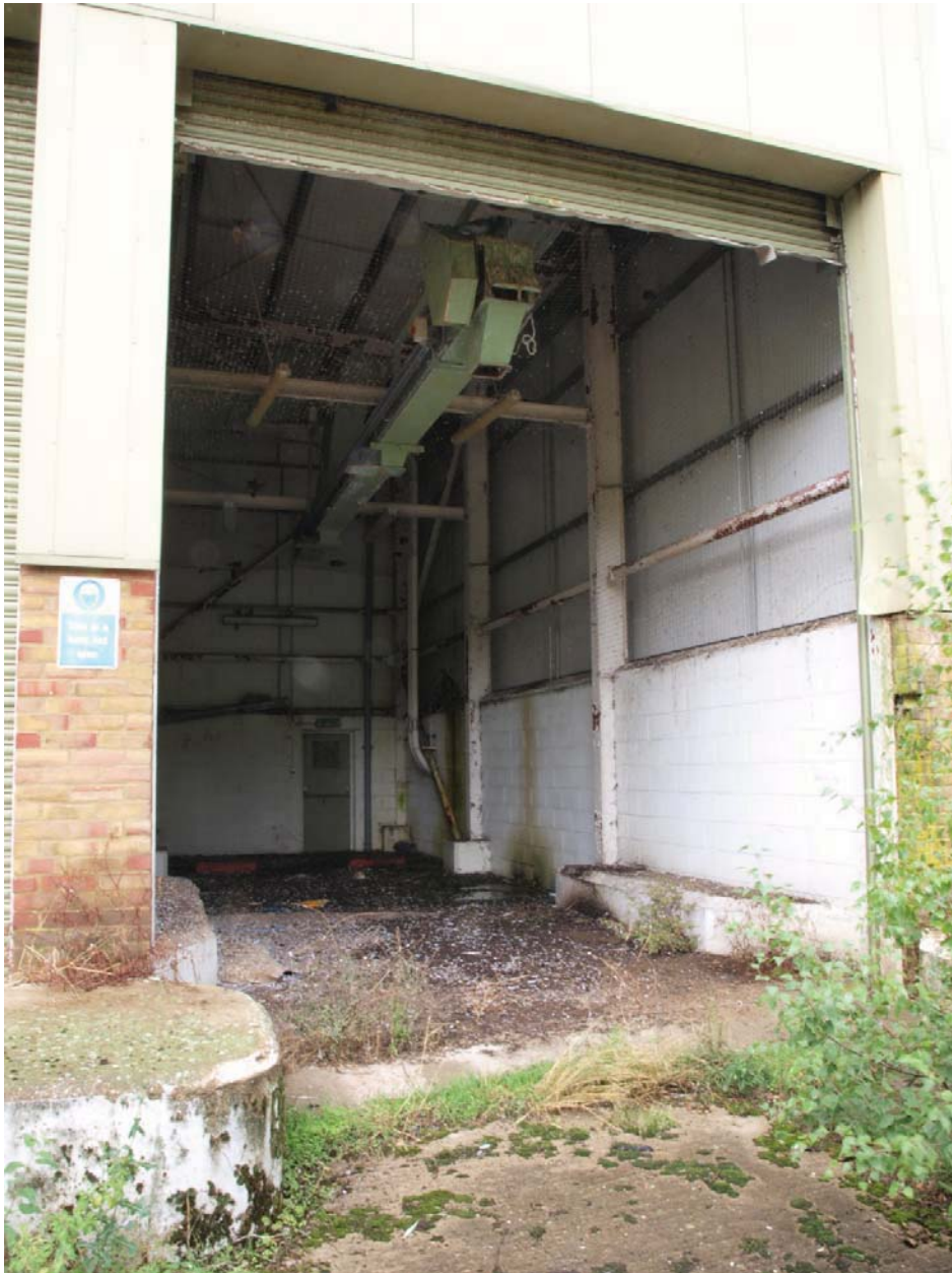
North loading bay and grain drops in the northern extension of the Mill (see Figure 2 for location), view to north-west
