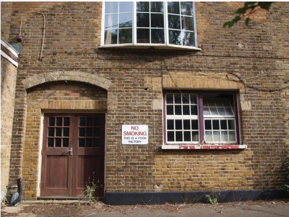
South elevation of Bakery (western extension of the Mill) with reduced entrance (left) and conversion of a former doorway into a window (see Figure 2 for location), view to north.
