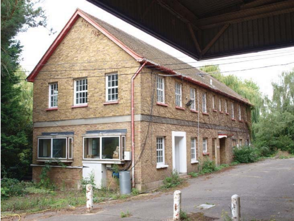
East (left) and north (right) elevations of the Administration Block (see Figure 2 for location). View to west-south-west.
