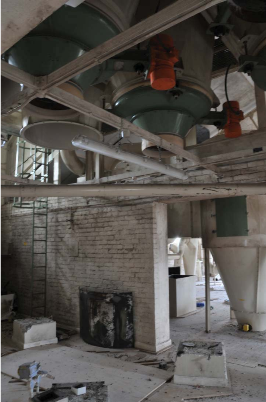
Brick wall on north side of second floor in the Mill's eastern extensions (see Figure 13 for location), view to north-east
