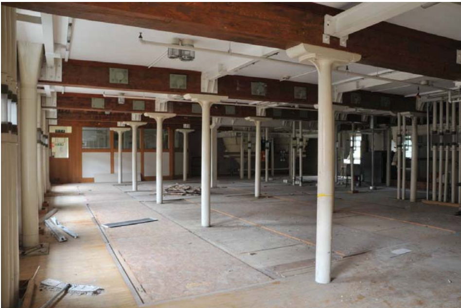
Original columns, first floor of Mill (see Figure 13 for location). View to north-west.
