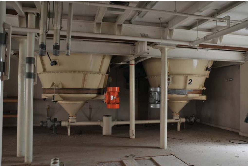
Grain hoppers in north-west corner, first floor, Mill (see Figure 13 for location).
