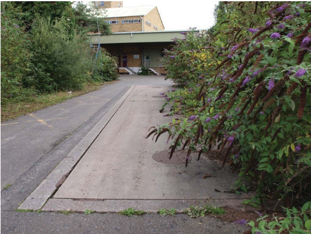
Northern most concrete weighbridge with centrally positioned man hole covers, looking north.
