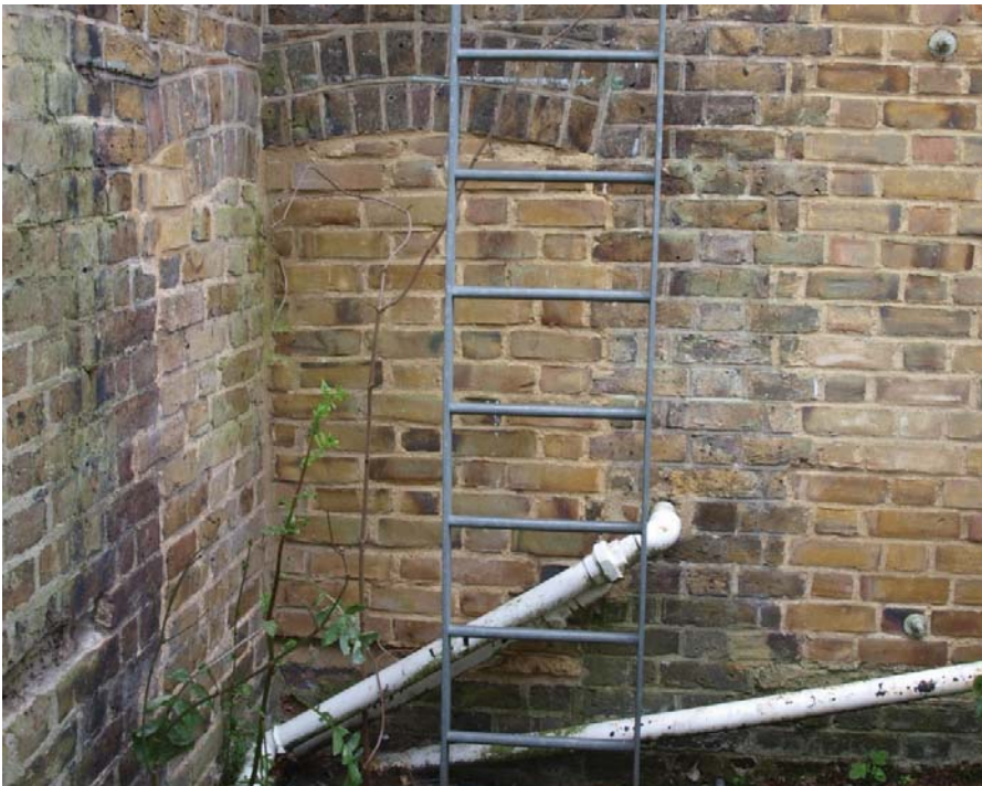
Infilled windows on west (left) and north (right) elevation of western extension of the Mill (see Figure 2 for location), view to south
