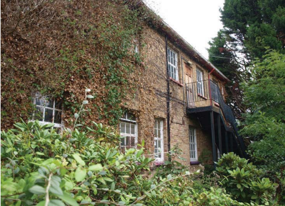
South Elevation of Administration Block to east (see Figure 2 for location). View to east-north-east.
