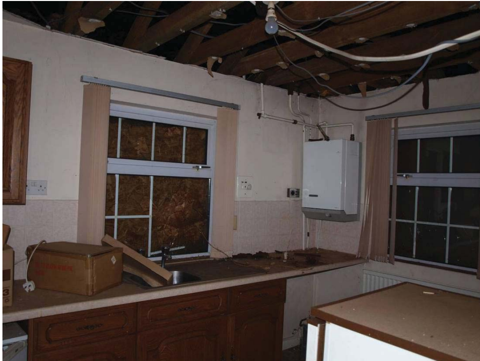
Ground floor kitchen, Kingsmill Cottage (see Figure 24 for location). View to north-west.
