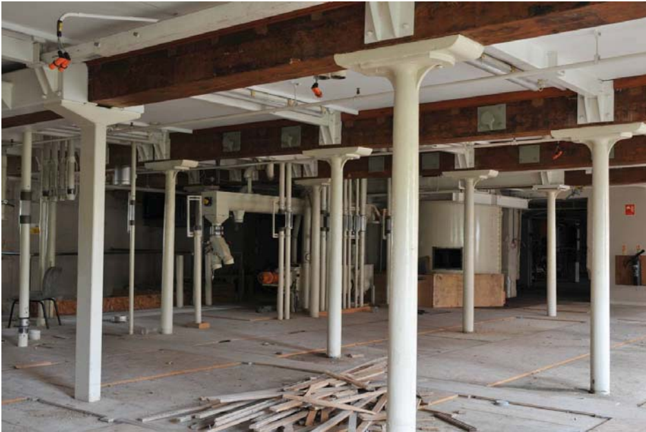
Combination of original and replaced columns, first floor, Mill (see Figure 13 for location). View to east-north-east.
