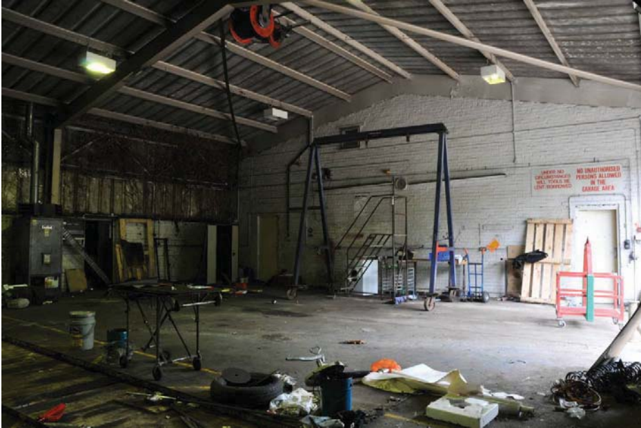
North end of Vehicle Workshop (see Figure 2 for location). View to south-east.
