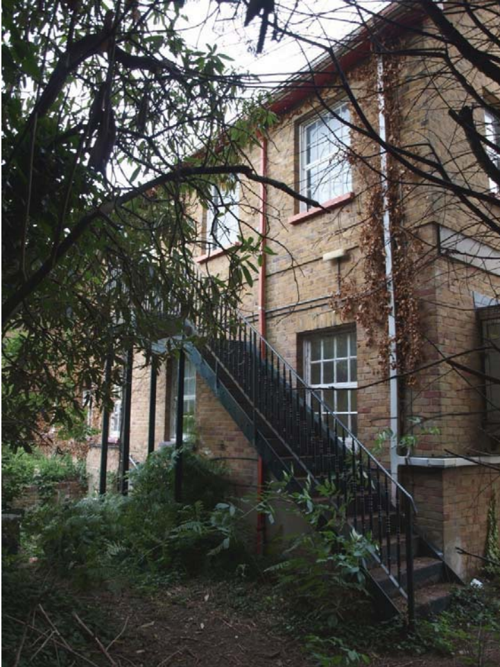
South elevation of Administration Block to east (see Figure 2 for location). View to north-west.
