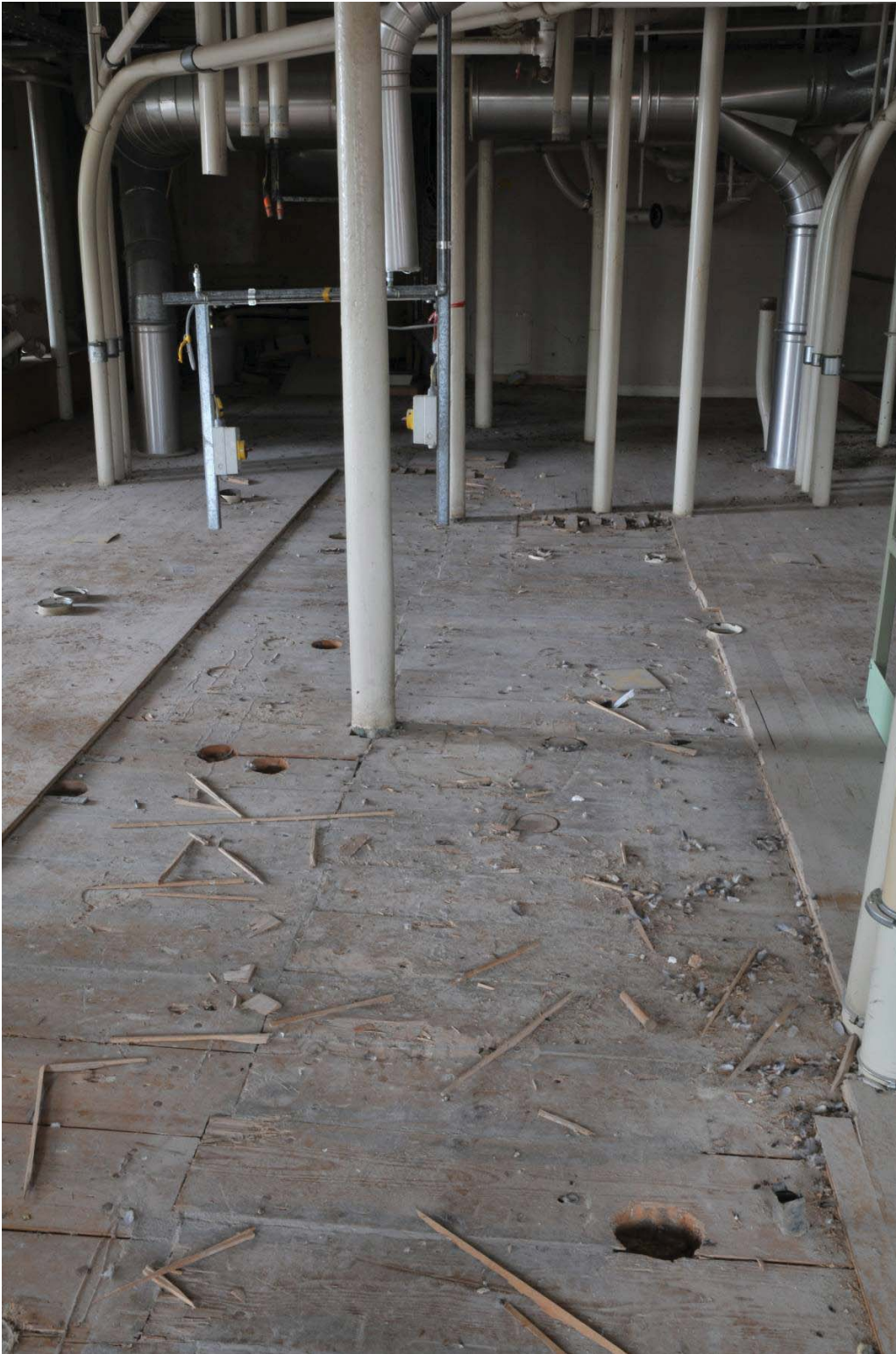
Replacement floorboards, second floor of Mill (see Figure 14 for location). View to north.
