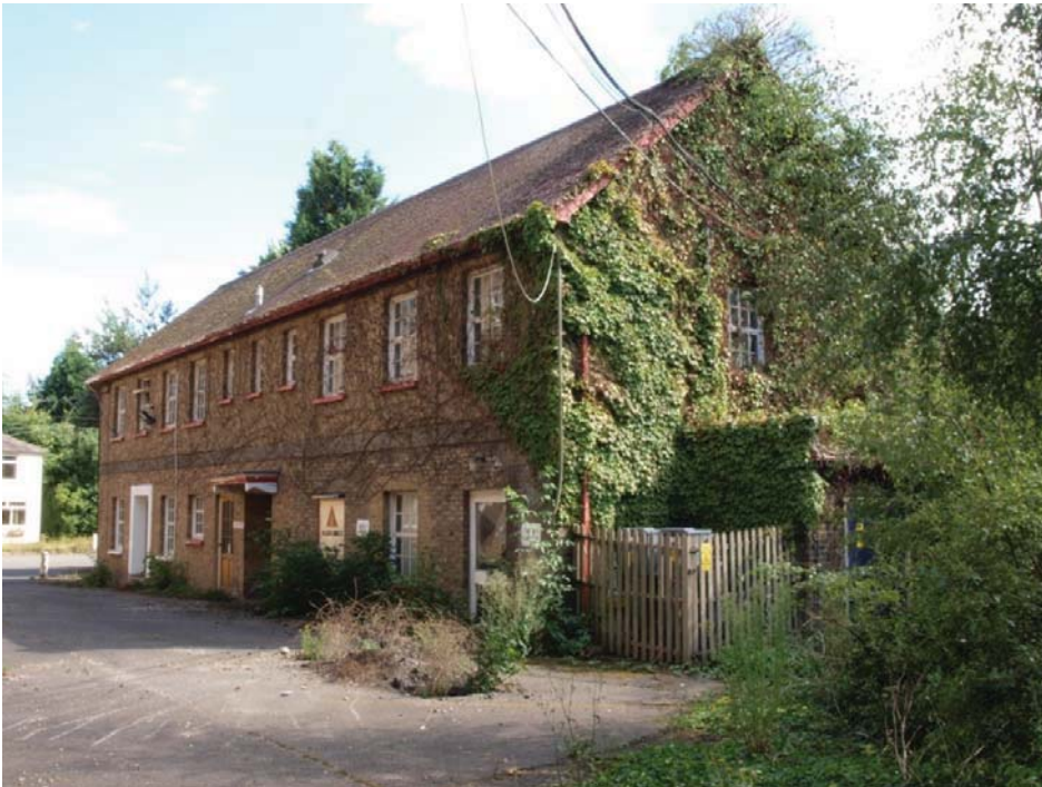
North Elevation of Administration Block (see Figure 2 for location). View to south-east.
