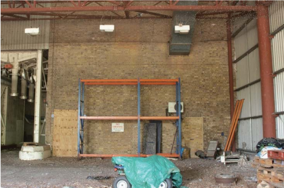
Northern part of the west elevation of the loading bay in the northern extension of the Mill (see Figure 2 for location), view to west
