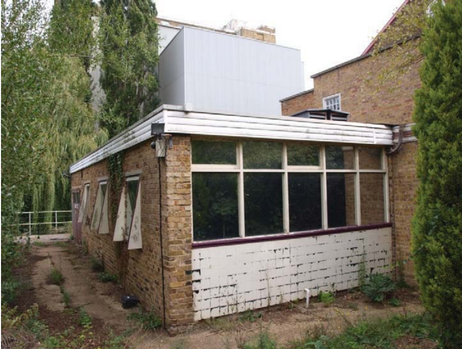
South elevation of the Laboratory, westernmost extension of the Mill (see Figure 2 for location), view to north-east
