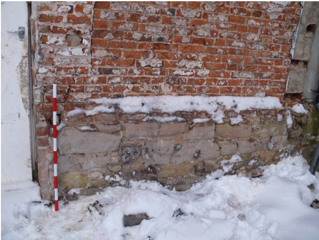
Plate 20. Detail of lower part of south facing elevation of eastern part of farmhouse. 1m scale.
