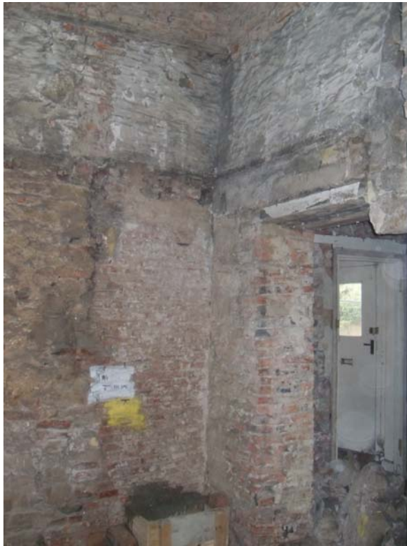
Plate 23. Detail of interior, brick rebuild in south-western corner of farmhouse. No scale.
