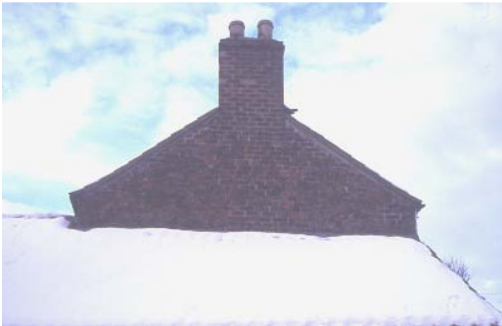
Plate 10. West facing elevation of upper part of gable end of farmhouse. No scale
