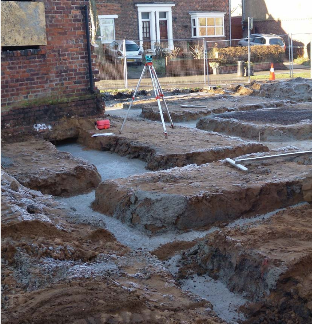
Figure 14 Network of new build footings, with north end of remaining buildings, looking north-west
