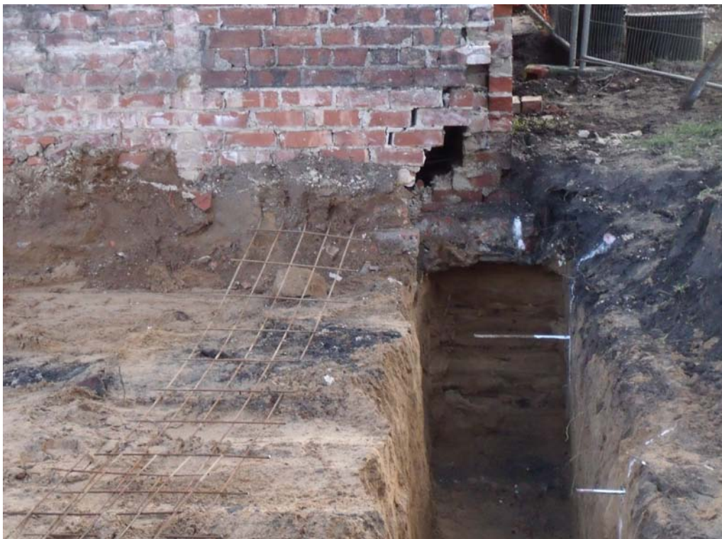
Figure 13 Westernmost element of new build footings adjacent to remaining building, looking south-east
