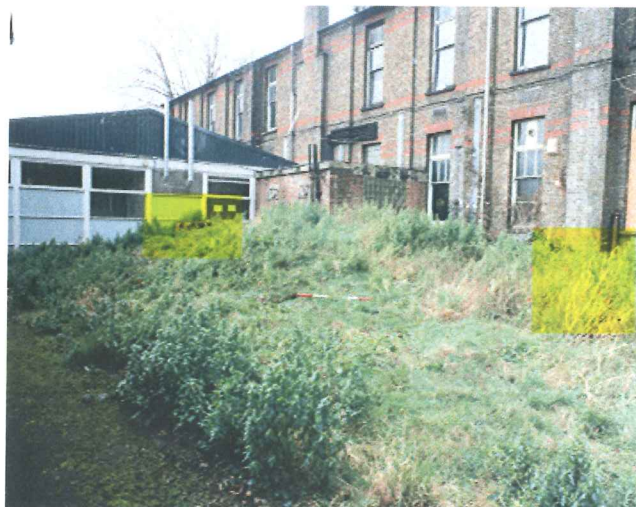
Plate 3 Exterior of shelter showing escape hatch (left) and area of entrance (right)
