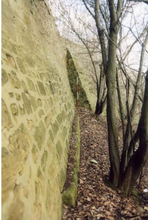
Plate 7. Stone underpinning of revetment wall. Northern end of Section 2, looking north-east (2m scale).
