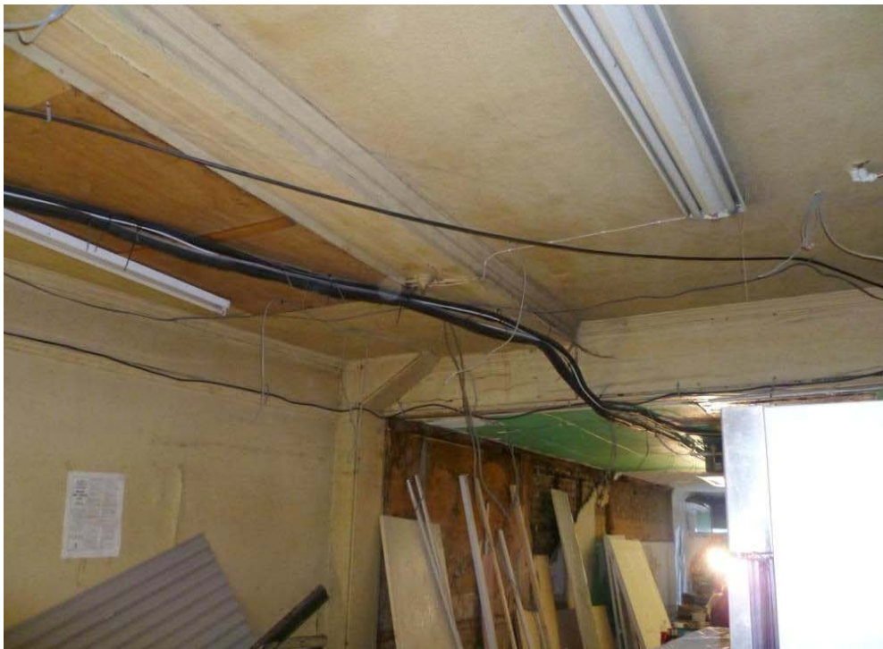
Plate 10. Looking east towards the shop front, showing cornice and east-west beam supporting the north wall of the rear extension (above) and north-south beam where the main rear wall once stood. The timber board (left) in the flat roof covers a skylight. (JM)
