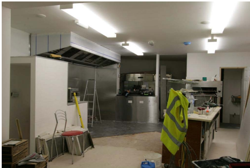
Plate 14. West end of the ground floor with a partially installed new kitchen (compare with Plate 12 before refurbishment). On the right of the far wall is the door to the toilet, in the centre the former door and window into the now enclosed yard and on the left the doorway to the basement with the staircase to the first floor and partition wall removed. (PCA)
