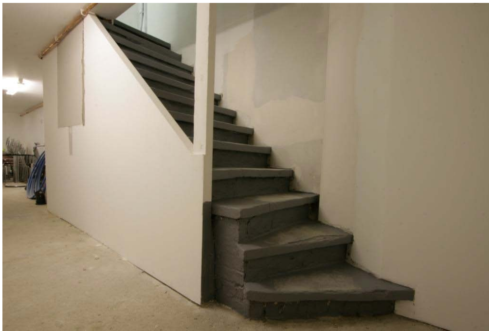
Plate 16. Stone and brick steps down to the basement after refurbishment with new side wall and replacement timber post. (PCA)
