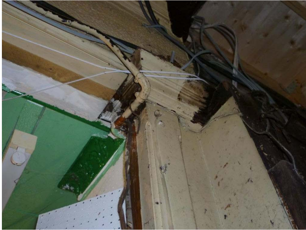
Plate 11. Cornice and chamfered pillar between the main building and rear extension. (JM)
