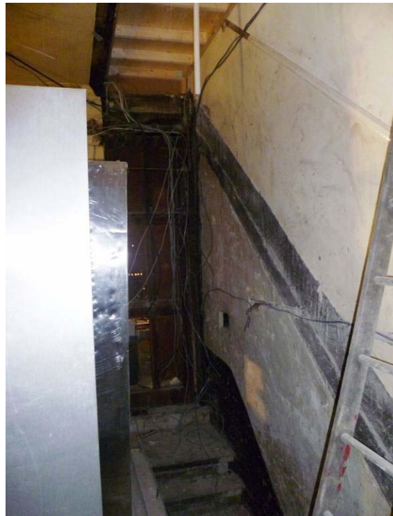
Plate 8. Stairs down to the basement with skirting board, dado and paintwork showing the original location of the stairs to the first floor. (JM)
