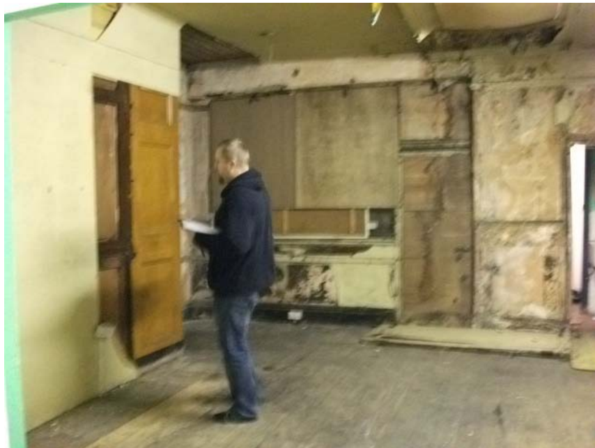
Plate 12. On left (south) is the timber panelled wall (now removed) of the staircase to the basement and first floor. In the centre is the boarded over original window (now removed) of the rear (west) extension, with the boarded over door (now removed) to the yard and on the right (north) the doorway to the toilet with a red tiled floor and Belfast sink. (N)
