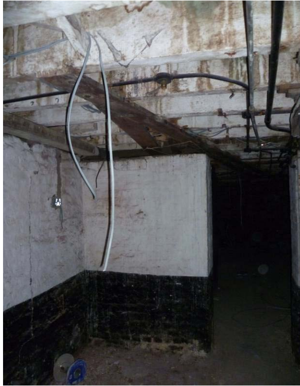
Plate 17. West end of basement from the foot of the steps showing north-south timber floor joists, on left north wall of the rear extension and the rear wall of the main building. (JM)
