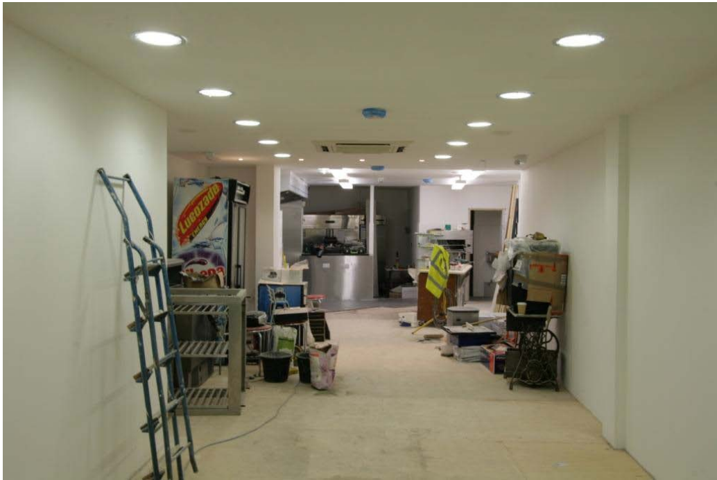
Plate 5. View of the refurbished ground floor with a new kitchen area at the far end (west) and a new corridor enclosing the staircase to the first floor on the left (south). (PCA)
