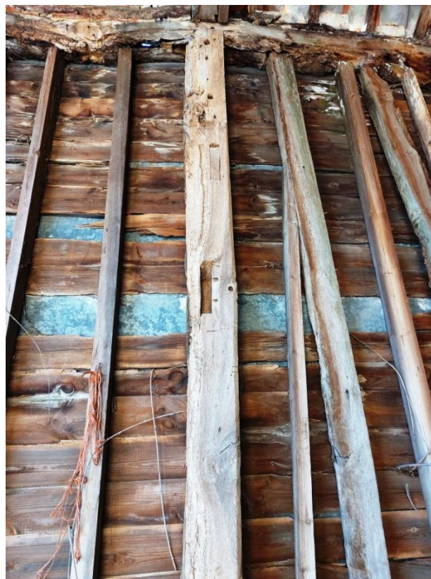
Plate 16. Vacant mortise and tenon joint on south wall storey post
