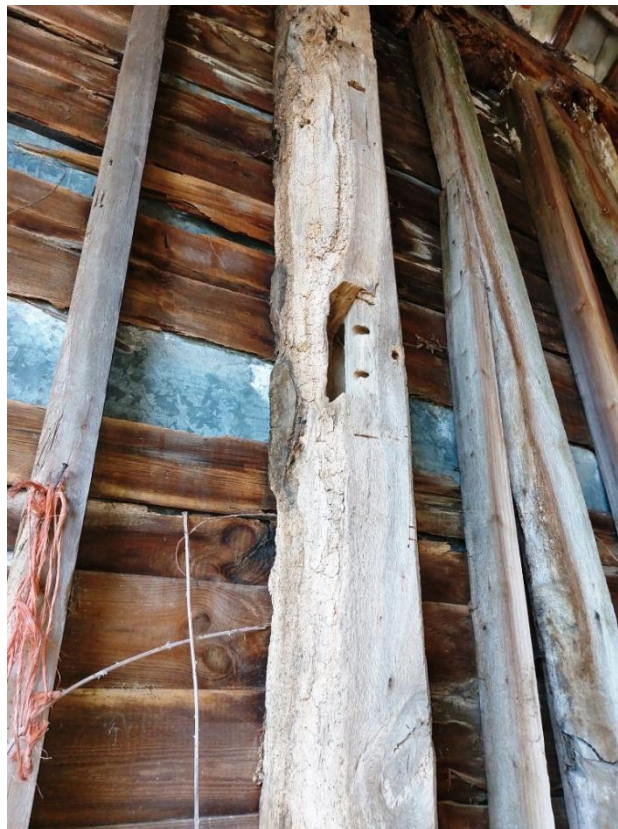
Plate 38. Vacant Tenon and Mortise joint on south wall (former arch brace joint)
