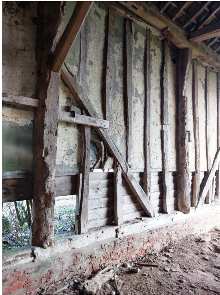
Plate 39. North wall interior posts with no vacant joints for arch braces
