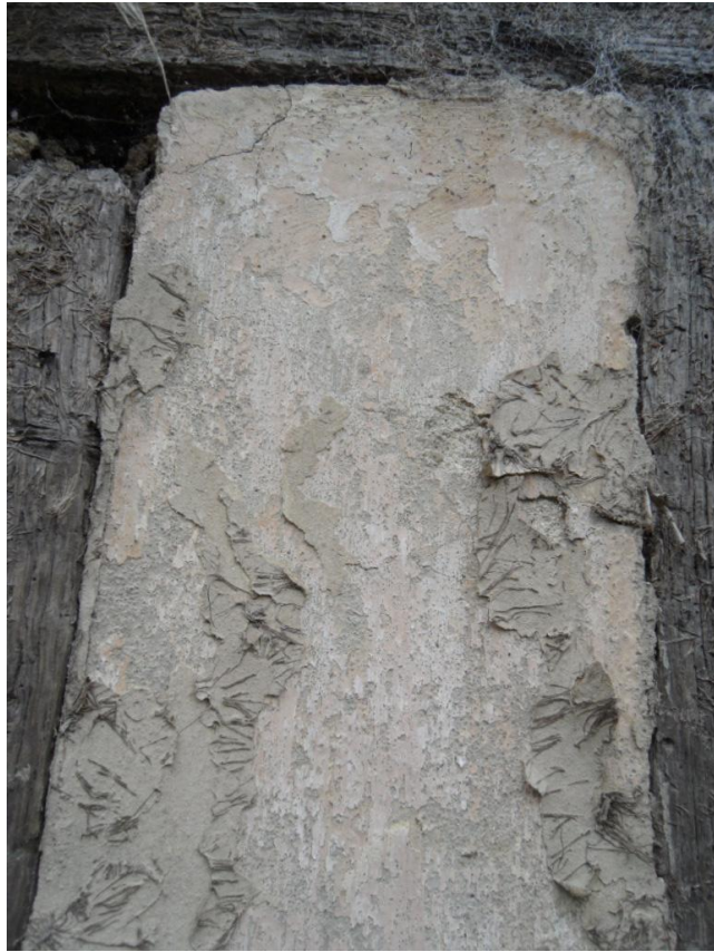
Plate 22. Original wall infill of plaster showing a primary paint surface-pinkish in colour, front elevation
